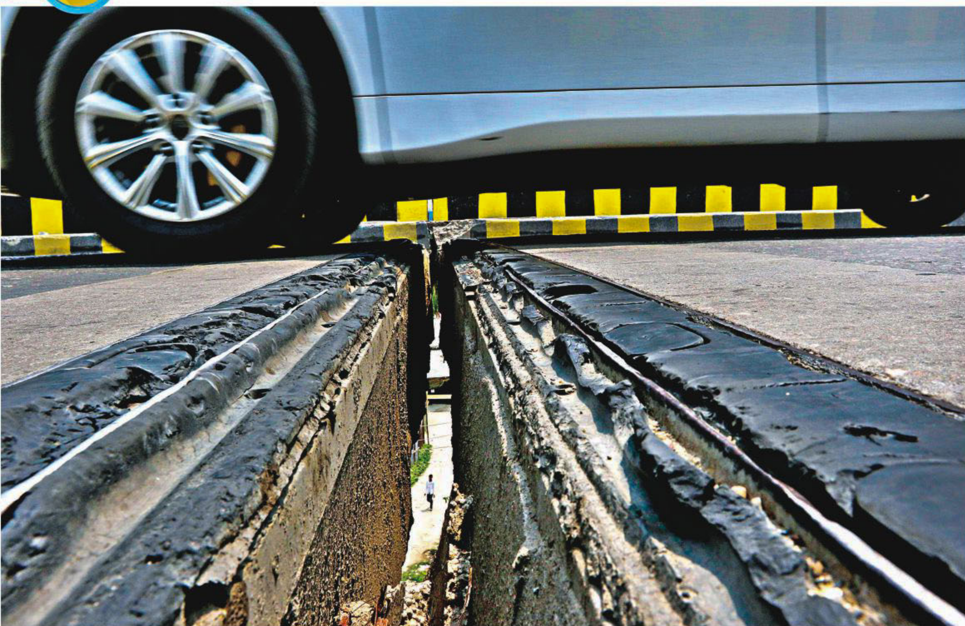
A car drives over a large crack on a lane of Sultana Kamal Bridge over Shitalakkhya River. Due to high traffic volume and lack of maintenance, the expansion joints have become damaged in at least three spots. The cracks have developed in such a scale that one can even see the road underneath. What's even scarier is that this situation is prevailing for over a year. The photo was taken at Demra on Friday.
