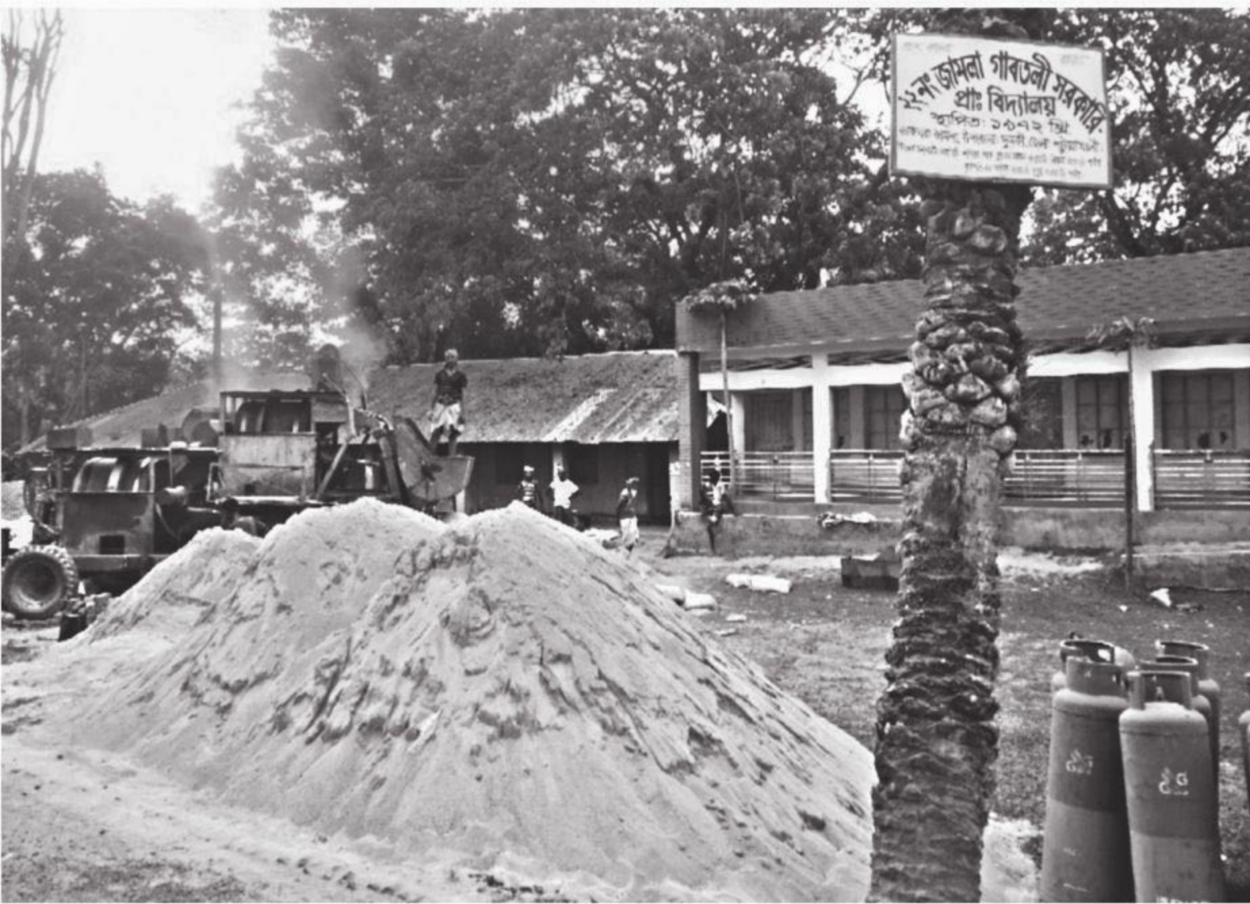
The school ground in Patuakhali's Dumki upazila has been filled with construction materials, including stone, sand, mixture machine, gas cylinders and bitumen.
