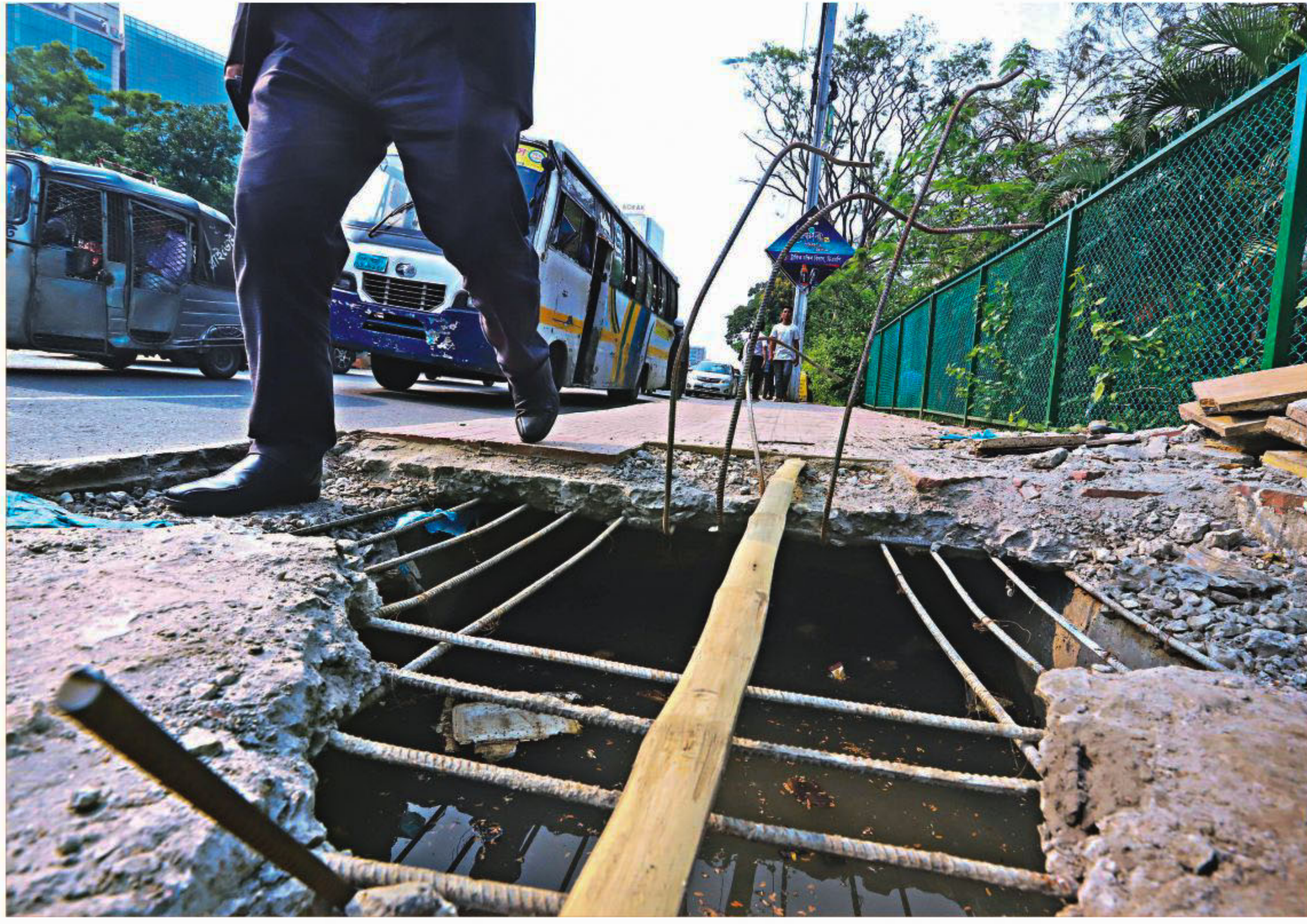
A pedestrian walks by a large hole on the footpath on the capital's major thoroughfare Kazi Nazrul Islam Avenue yesterday afternoon. A momentary lapse and a fall into the drain might completely ruin one's day or cause life-threatening injuries.
