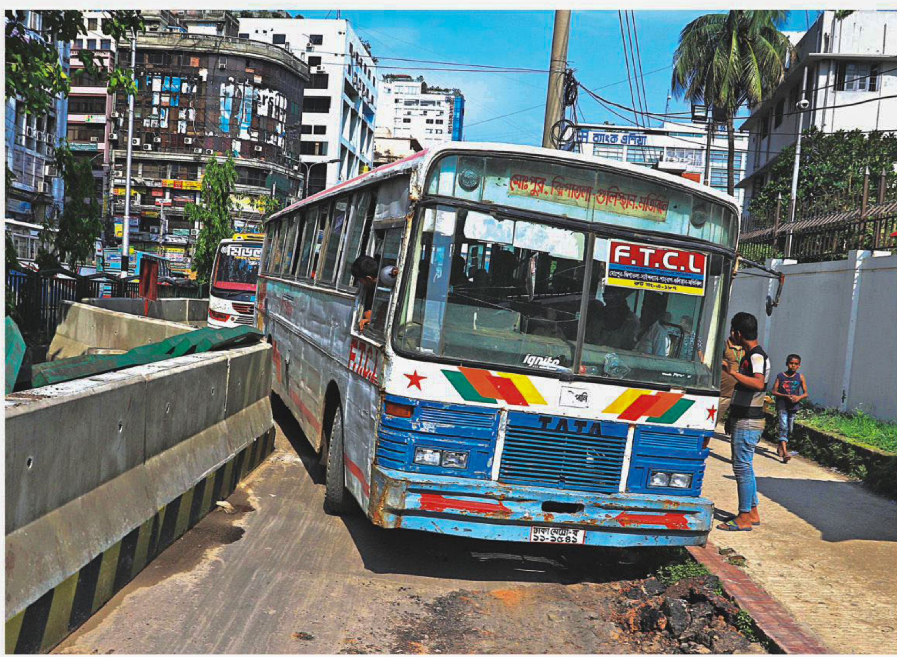
A bus almost gets on the footpath while trying to maneuver through the capital's Topkhana Road -- that has been significantly narrowed due to concrete road dividers placed as part of construction for the metro rail. The photo was taken yesterday.
