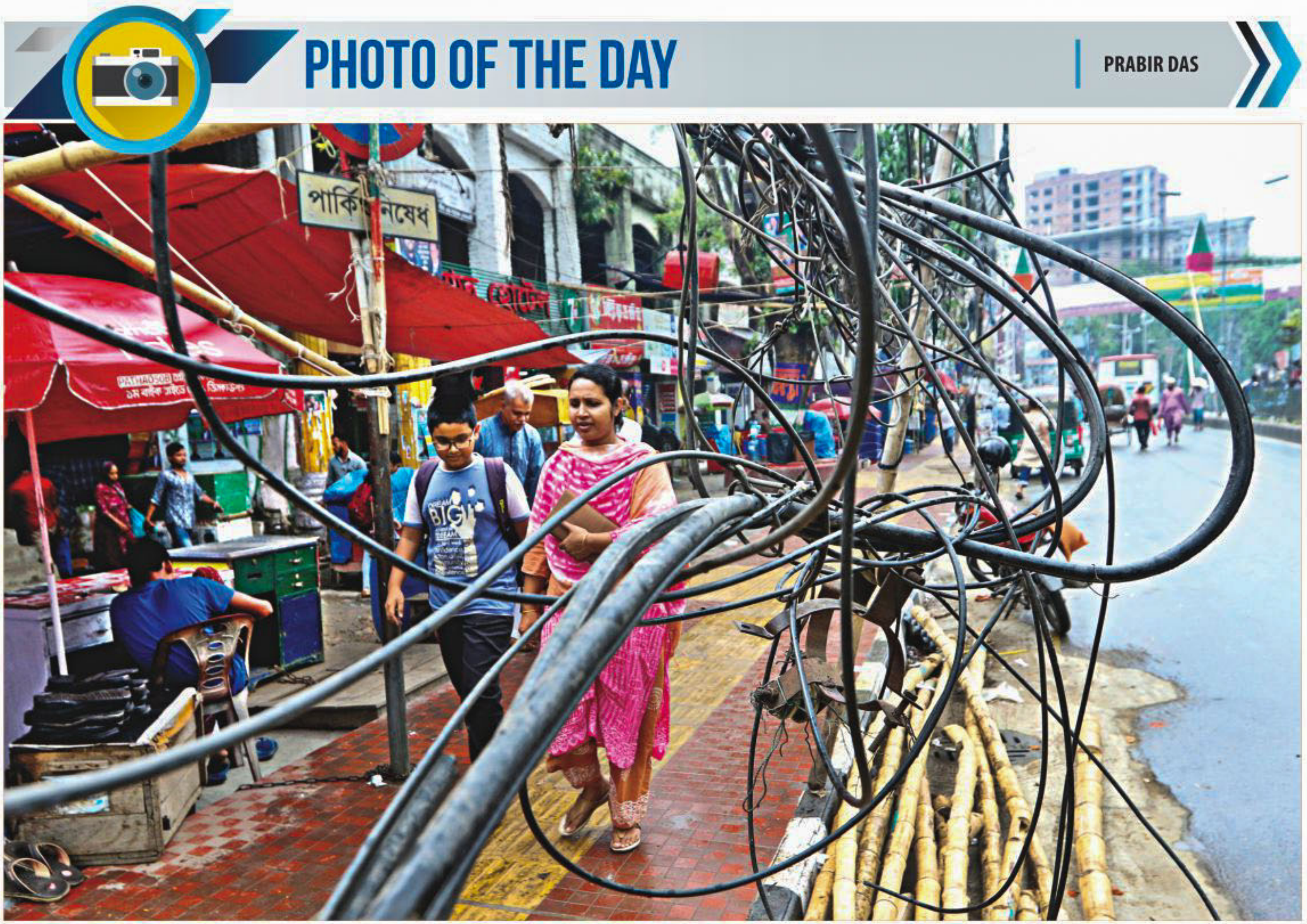
A tangle of cables -- including electrical lines -- hangs dangerously low on a footpath in front of Mohammadpur Town Hall Market. Locals say these have been in this condition for weeks, not only obstructing foot-traffic but also posing risks.
