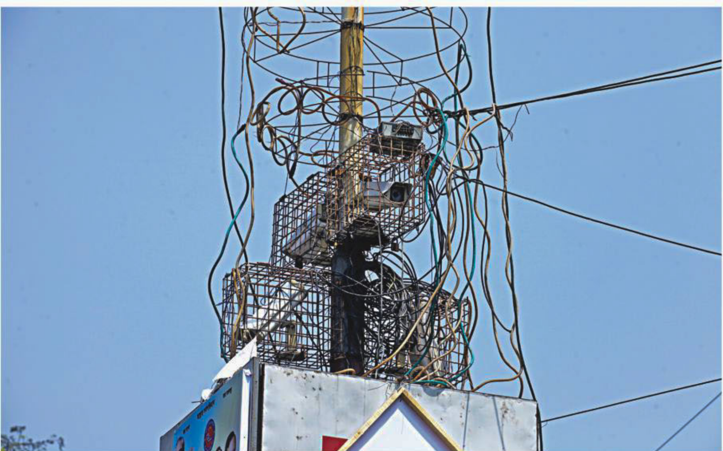
Tangled cables obstruct CCTV surveillance of Sylhet city's Chauhatta point. The Sylhet City Corporation had installed CCTV cameras in some key areas of the city to boost security, but poor maintenance of the devices is making the system less effective. The photo was taken on Sunday.
