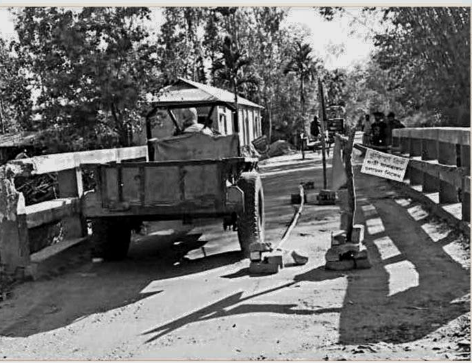
The authorities concerned have put up a warning sign on the risky bridge across Golakata canal in Gaibandha's Sundarganj upazila, asking vehicles not to use the structure.
