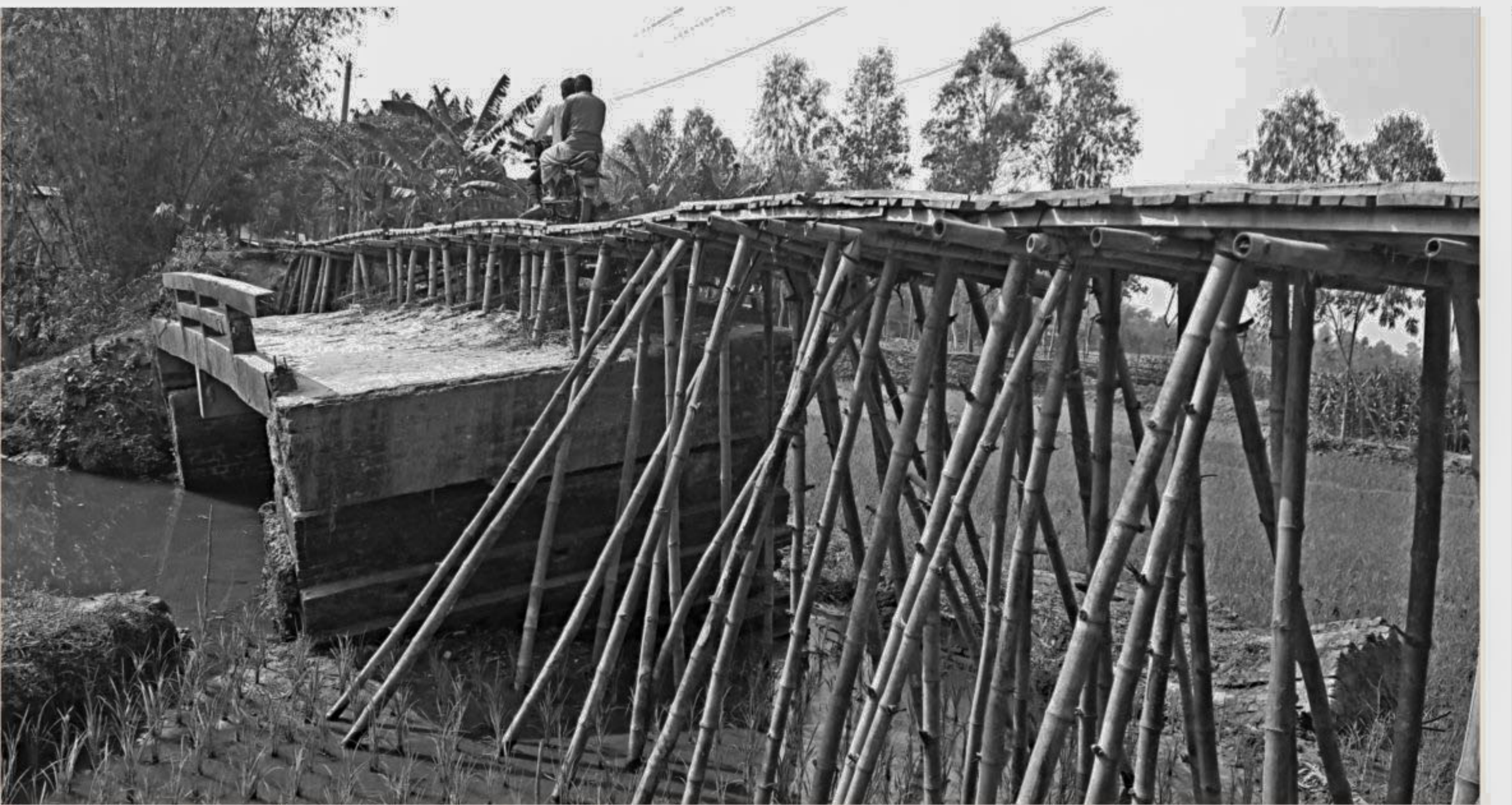
A recent photo of the wobbly makeshift bridge that locals made on Kakina-Aminganj road after the original concrete bridge and its approach roads were damaged during floods in 2017.
