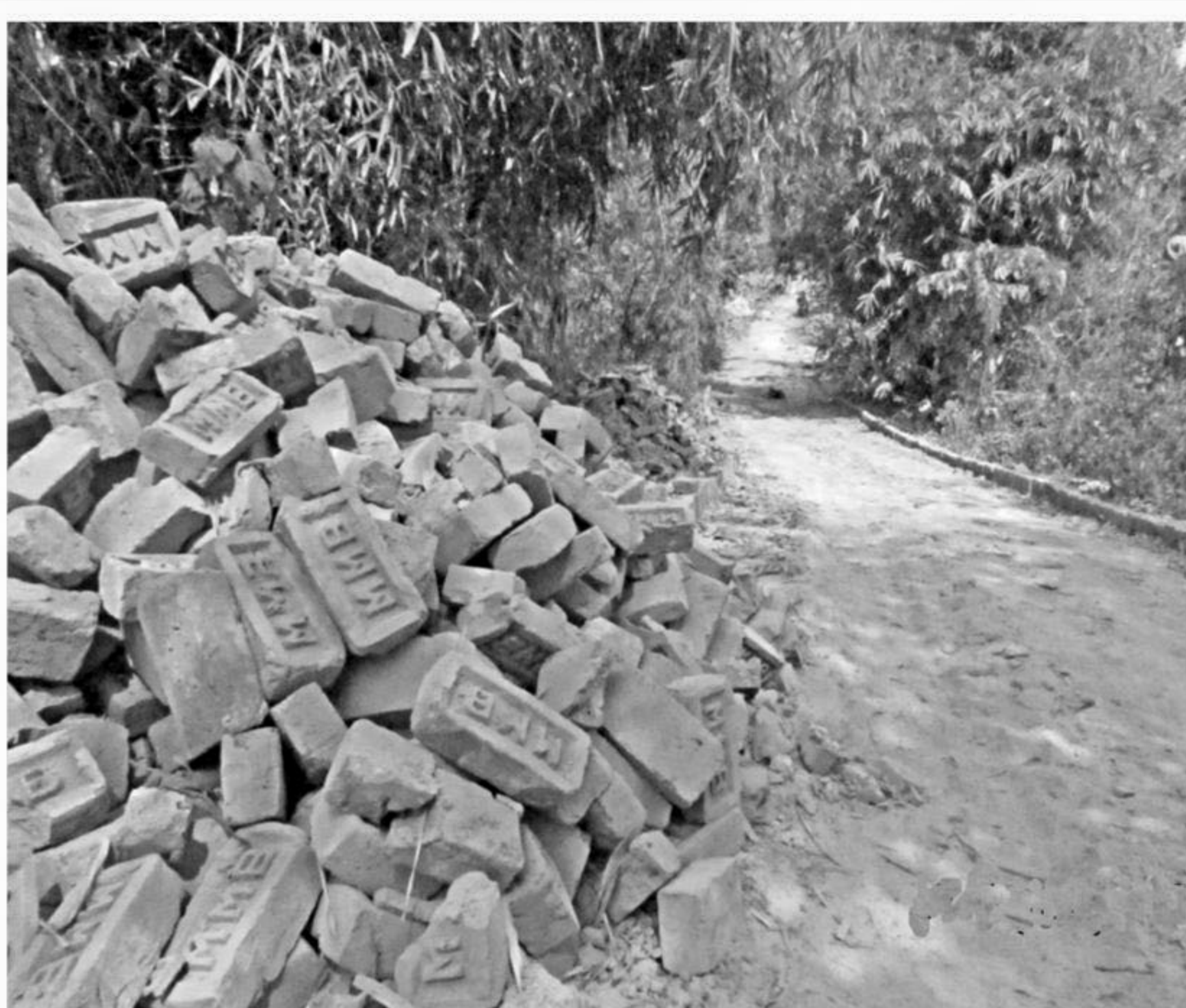
Construction of this half a kilometre road in Rangapanichhara area under Khagrachhari Sadar upazila is going on, using such low quality bricks.
