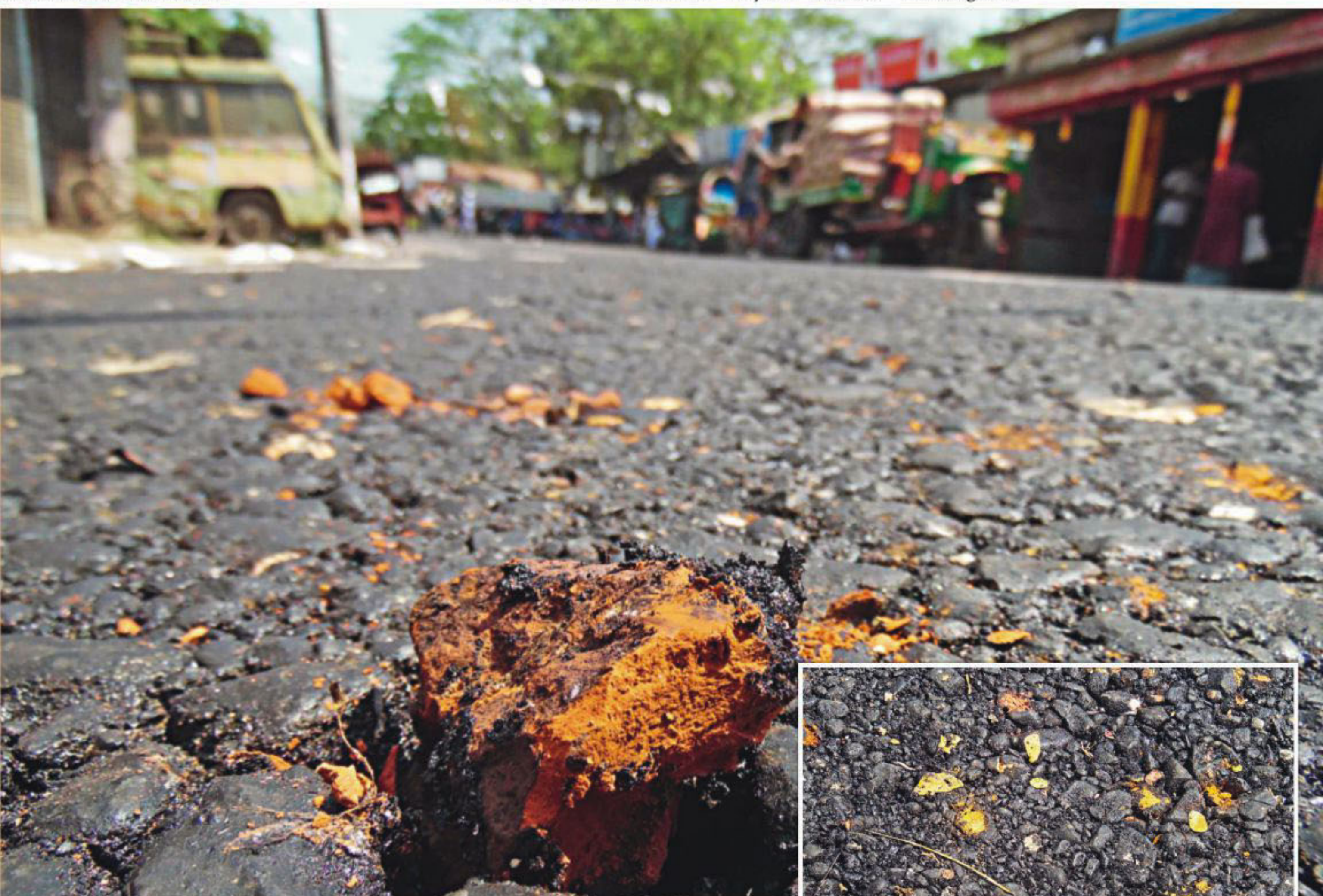
Brickbats, used in road construction, get exposed days after completion of carpeting at Rajapur Baipasmore in Jhalakathi, bearing testimony to the poor quality work.
