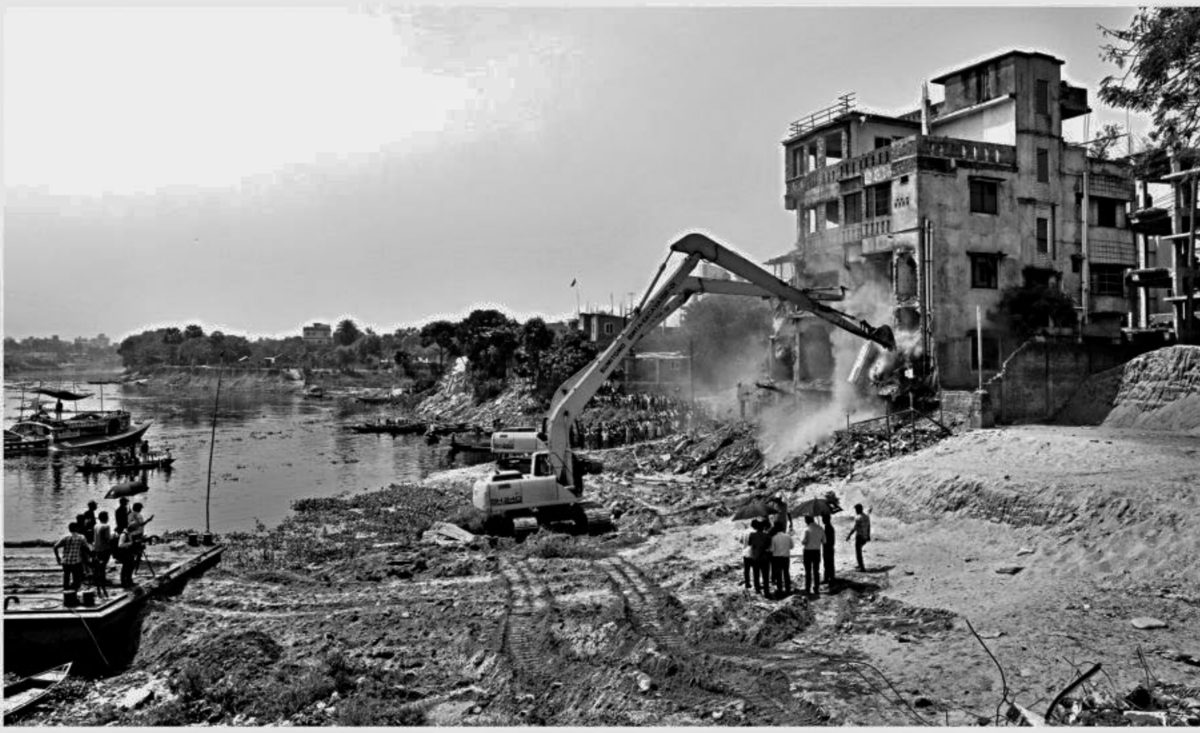
Authorities are demolishing illegal structures along the bank of Turag river in Savar, on the outskirts of the capital. The photo was taken yesterday.
