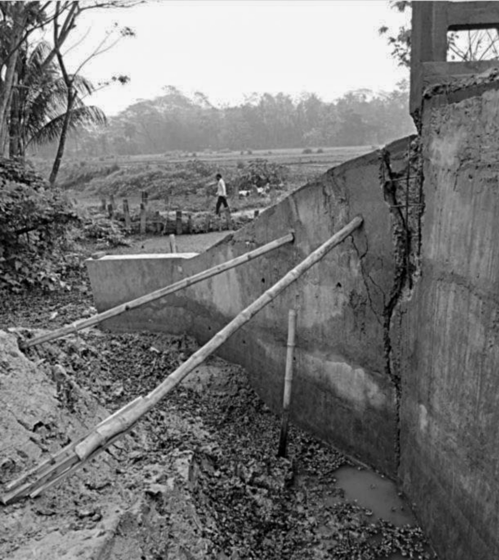
Bamboos are used to protect the cracked portion of the newly built culvert at Kuripaika village in Patuakhali Sadar upazila.
