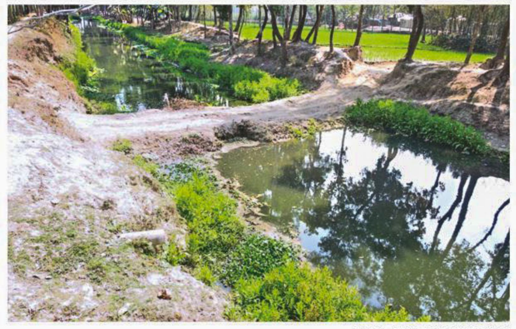
Another earthen road across the canal, only 300 metres from the above one. PHOTO: EAM ASADUZZAMAN
