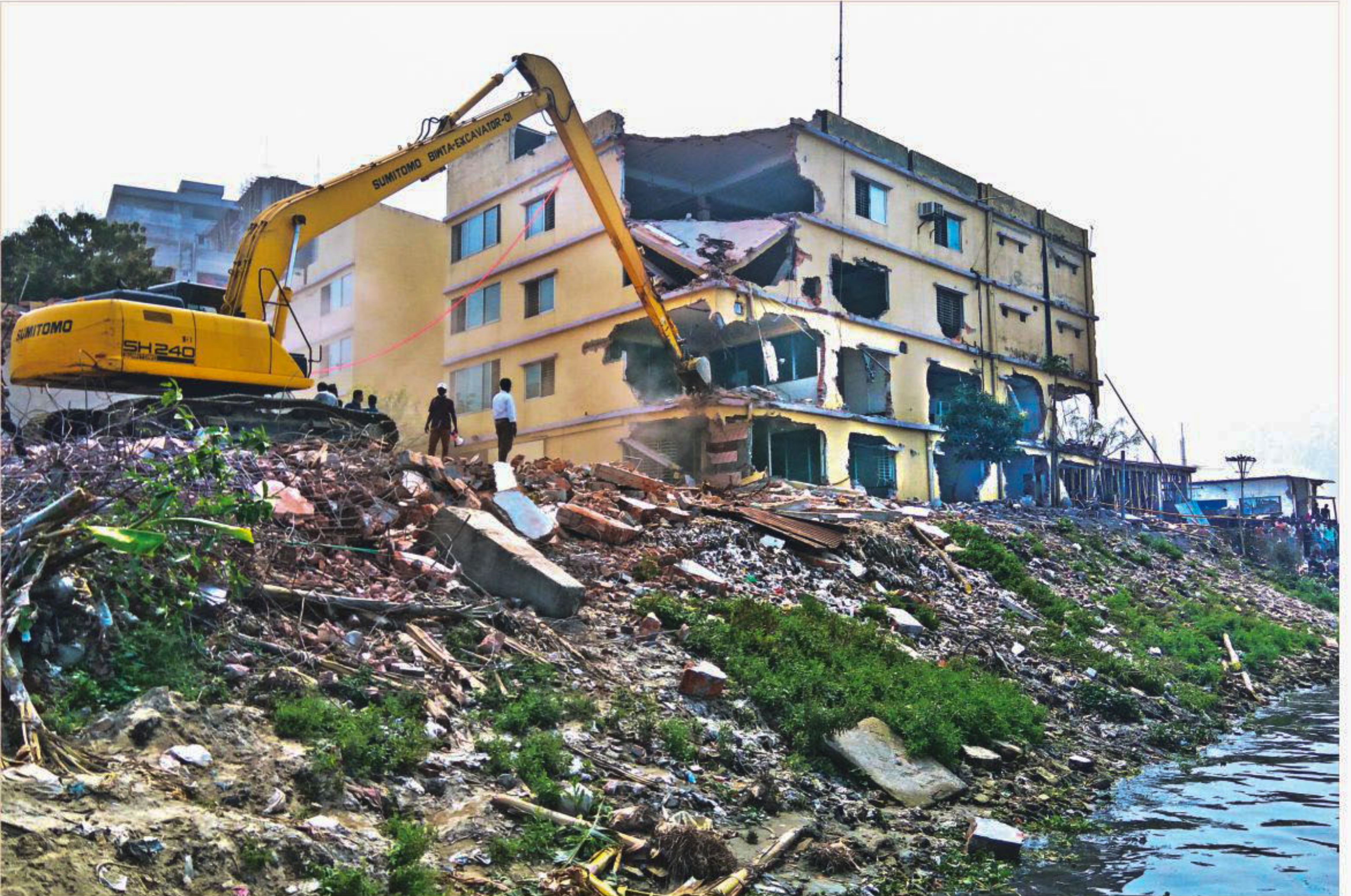
Bangladesh Inland Water Transport Authority yesterday knocked down some 57 structures as part of their on-going drive against illegal establishments along the Buriganga and Turag rivers. A total of 174 structures have been knocked down so far in the second phase of the drive which will be continued for seven more working days. This photo was taken at Dhaka Uddan Housing near Mohammadpur beribadh. PHOTO: RASHED SHUMON
