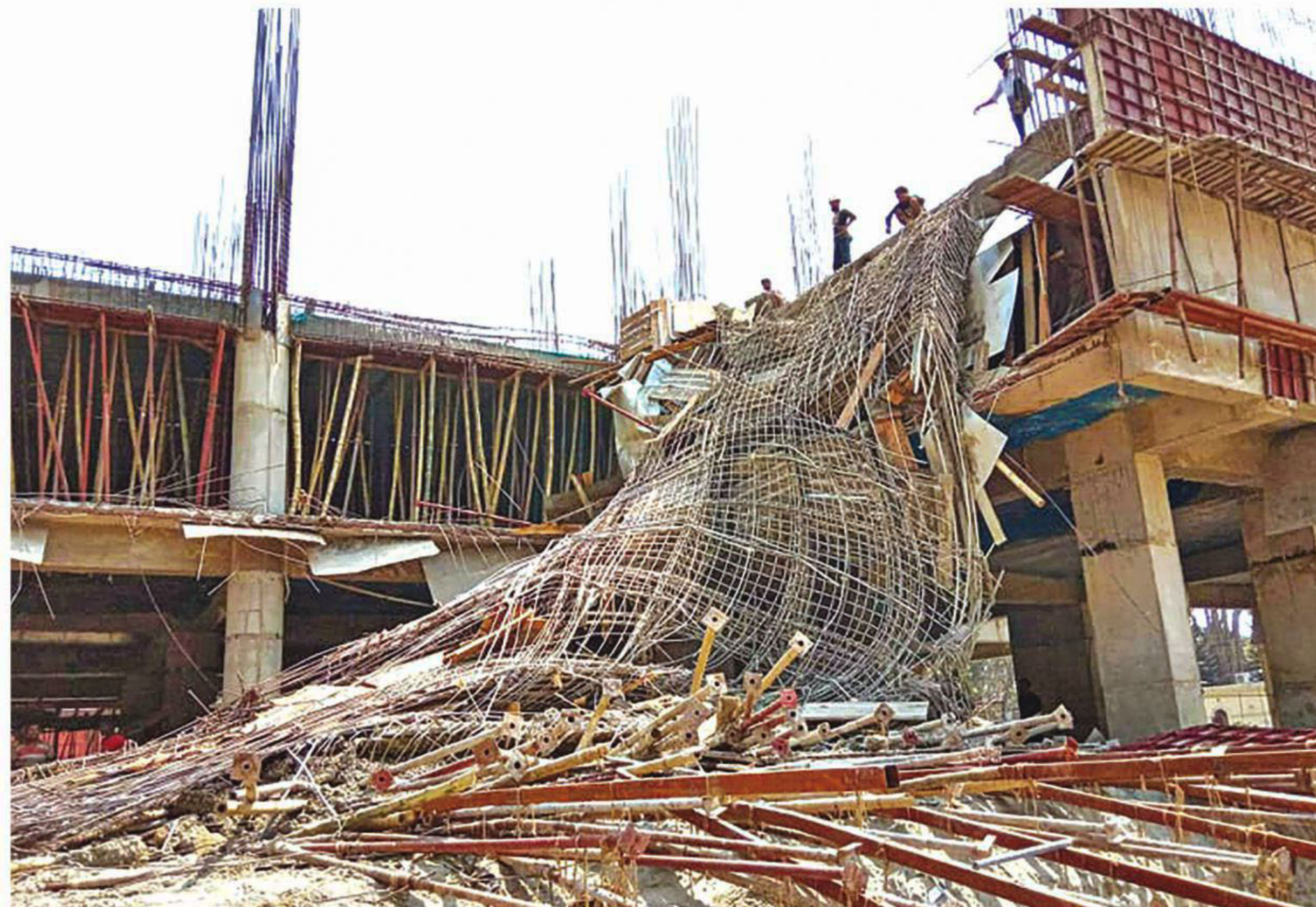
Construction workers look at the collapsed portion of an under-construction building on the campus of Tangail's Mawlana Bhashani Science and Technology University yesterday. The incident left at least 18 workers injured.
