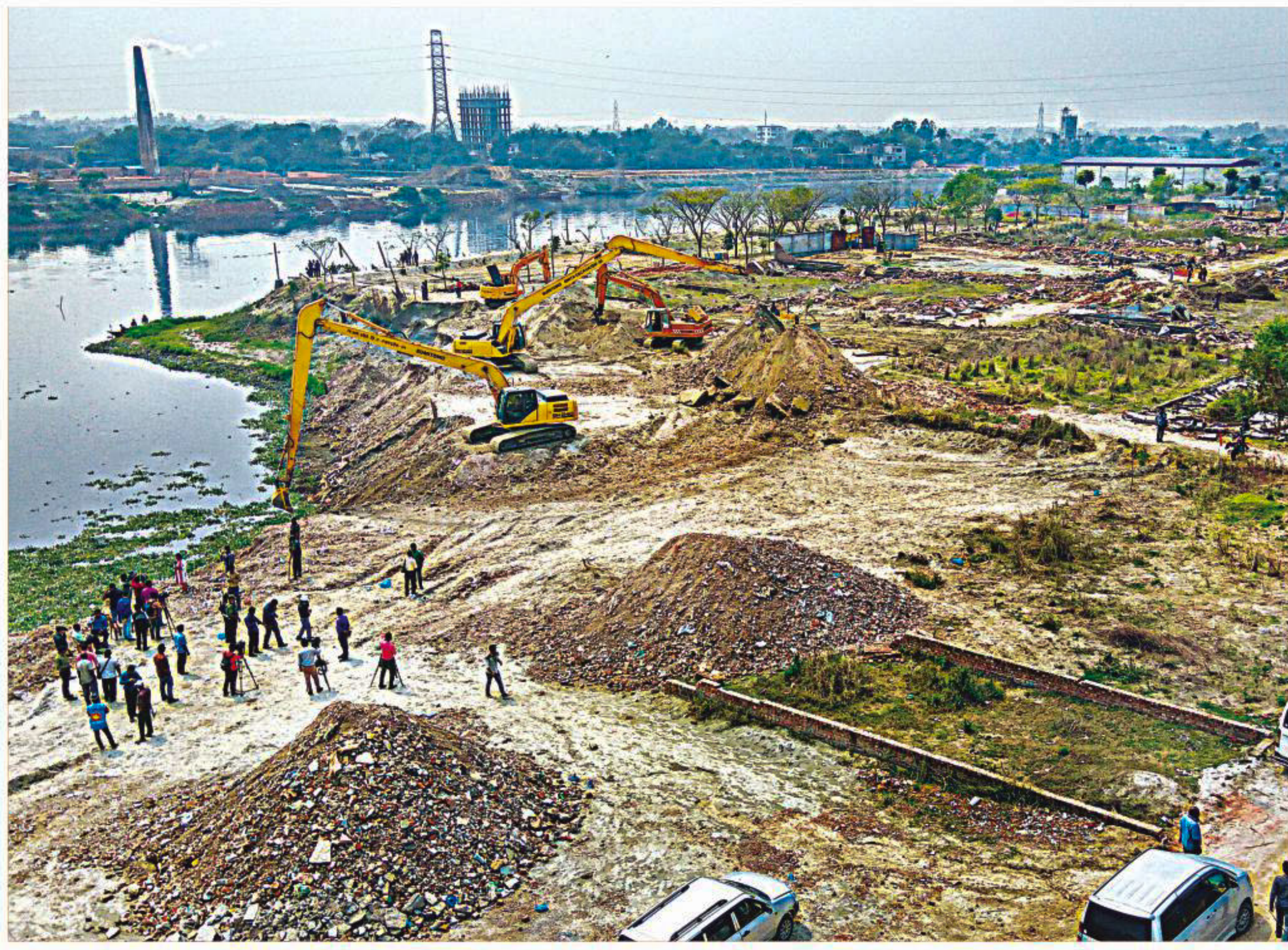
Excavators of Bangladesh Inland Water Transport Authority working on reclaiming a large part of the Buriganga river illegally filled-up by a real estate company in Bosila area of the capital. PHOTO: RASHED SHUMON
