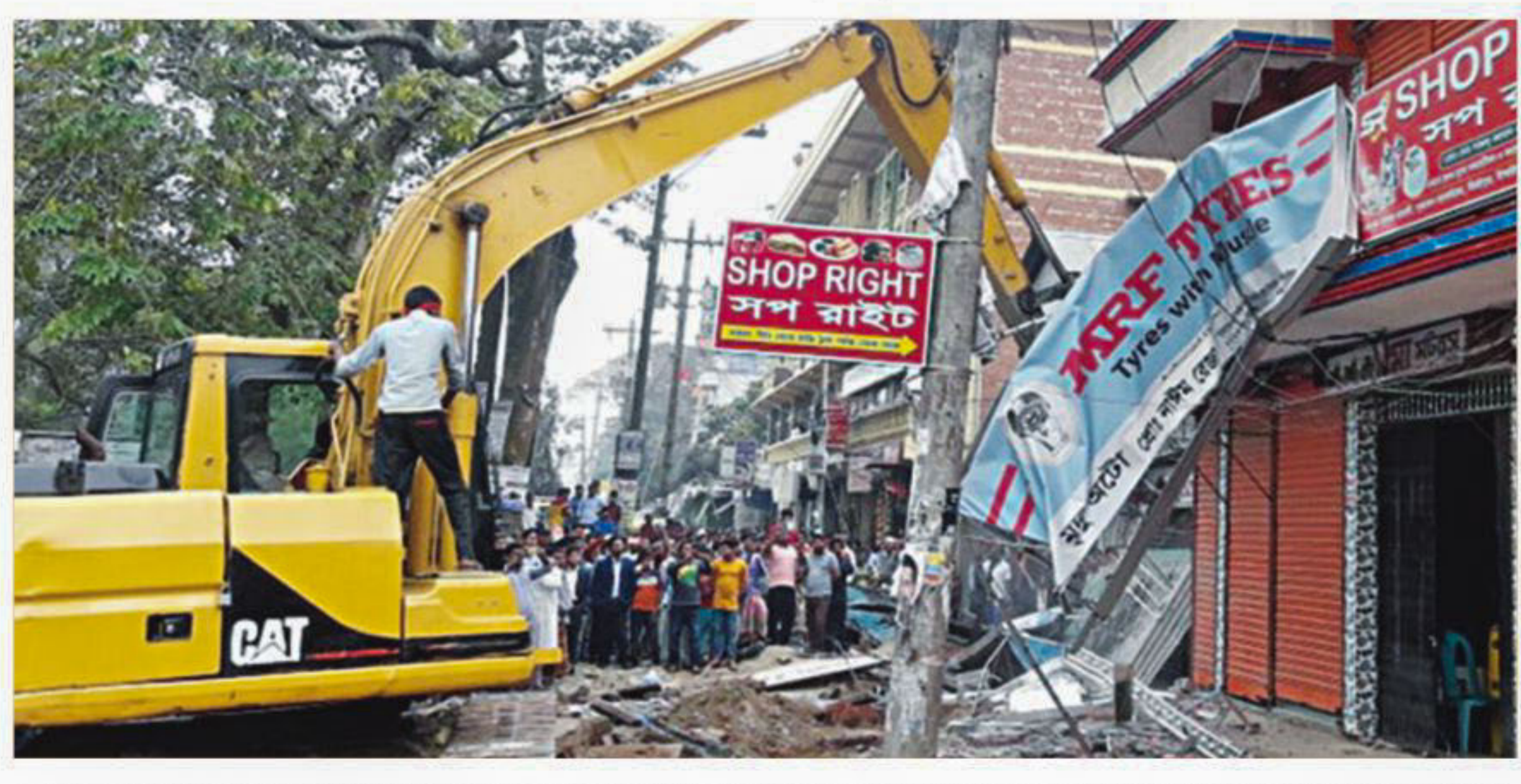
A bulldozer goes into operation as the Roads and Highways Department (RHD) conducts a drive yesterday to remove over 200 illegal structures in Old Bus Stand area of Mirzapur upazila in Tangail. PHOTO: STAR
