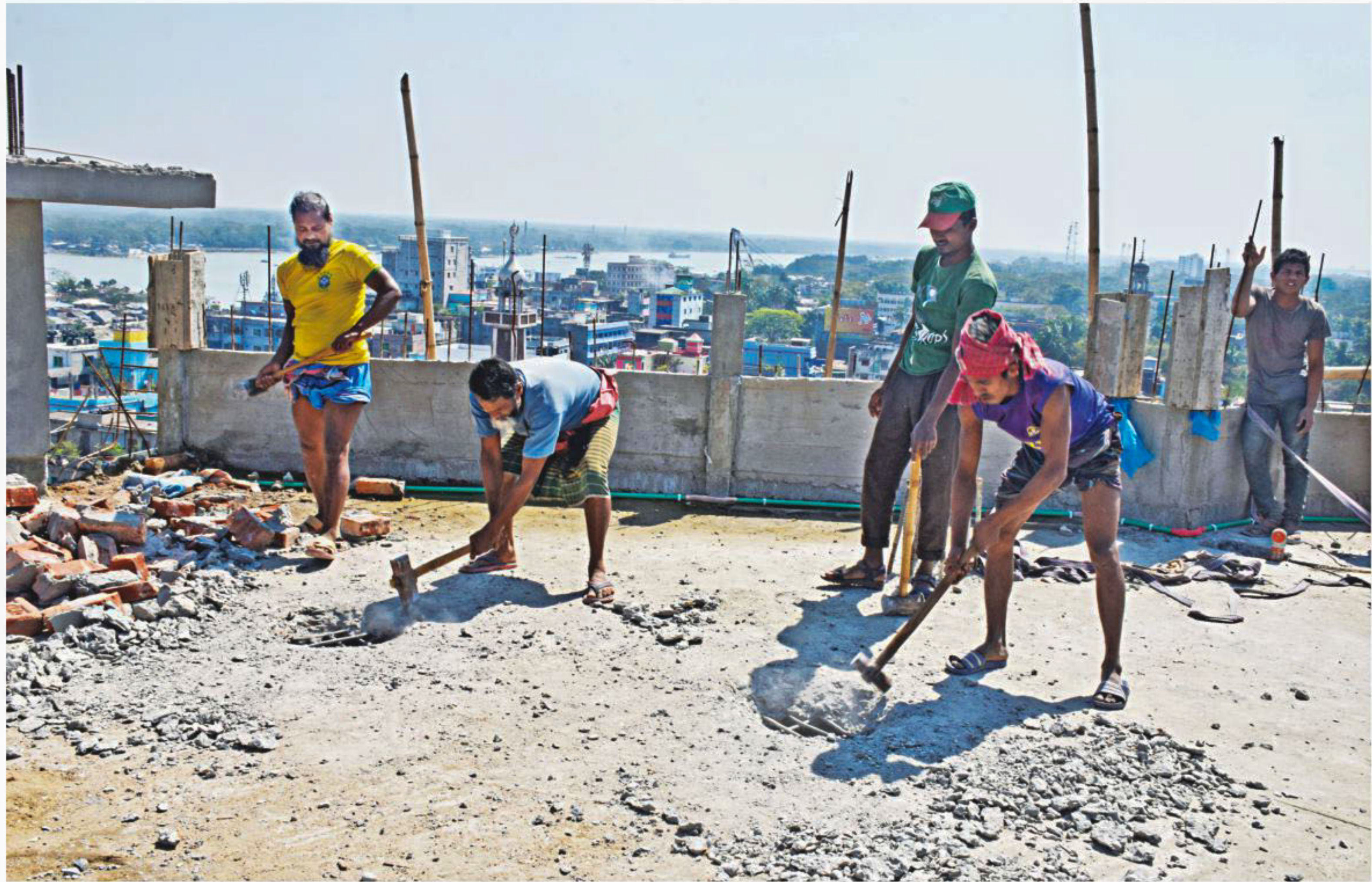
Barishal City Corporation starts demolishing illegally extended floors of an 11-storey building in Line Road area yesterday.
