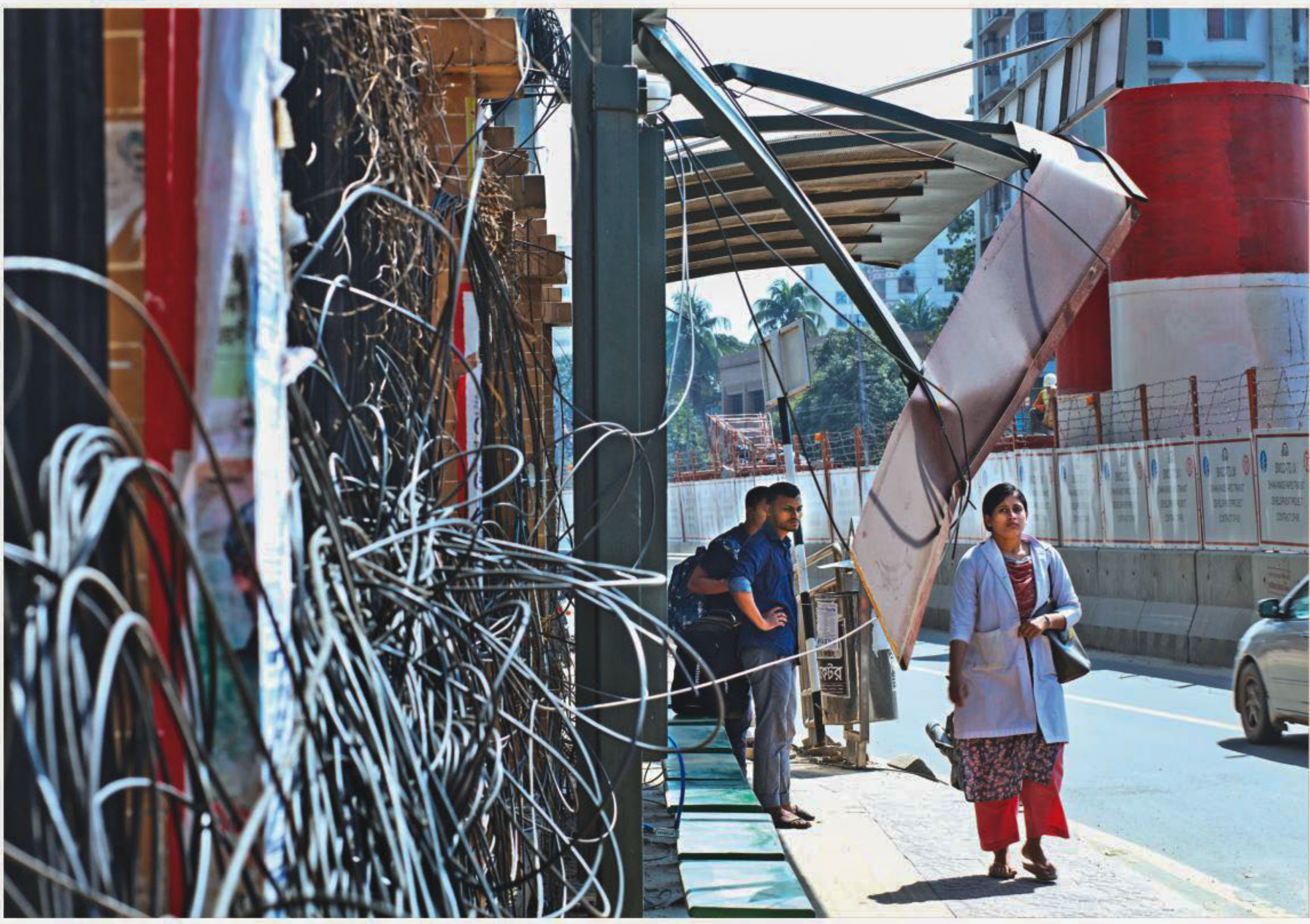
The shade over the roadside bench hangs loosely from its frame and may hurt pedestrians any moment. The picture was taken yesterday near Banglamotor intersection.
