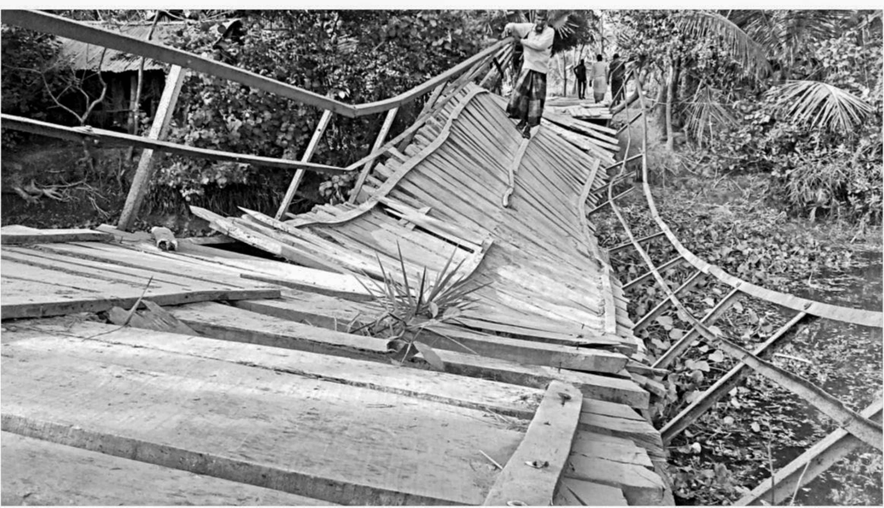
A man takes a risky walk on the awfully dilapidated iron bridge on the Kunimara canal in Kalapara upazila of Patuakhali. Around 30 thousand people of nearby villages are badly suffering as the authorities concerned have failed to replace the unusable structure. PHOTO: SOHRAB HOSSAIN
