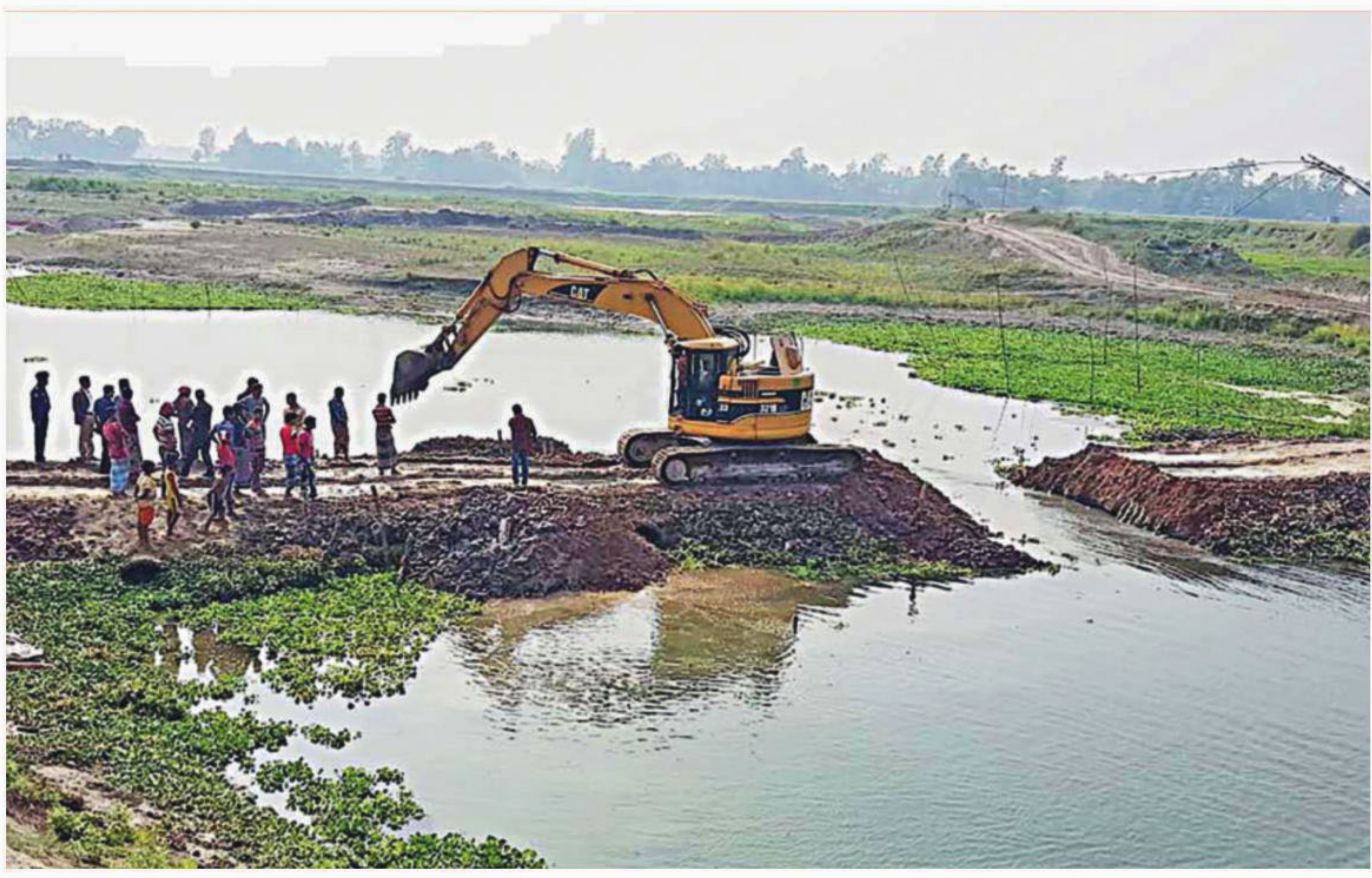
Mirzapur upazila administration demolishes one of the three roads, built illegally by an influential quarter across the Louhajang river in Bohuria area, for movement of earth-laden trucks to nearby brick kilns.
