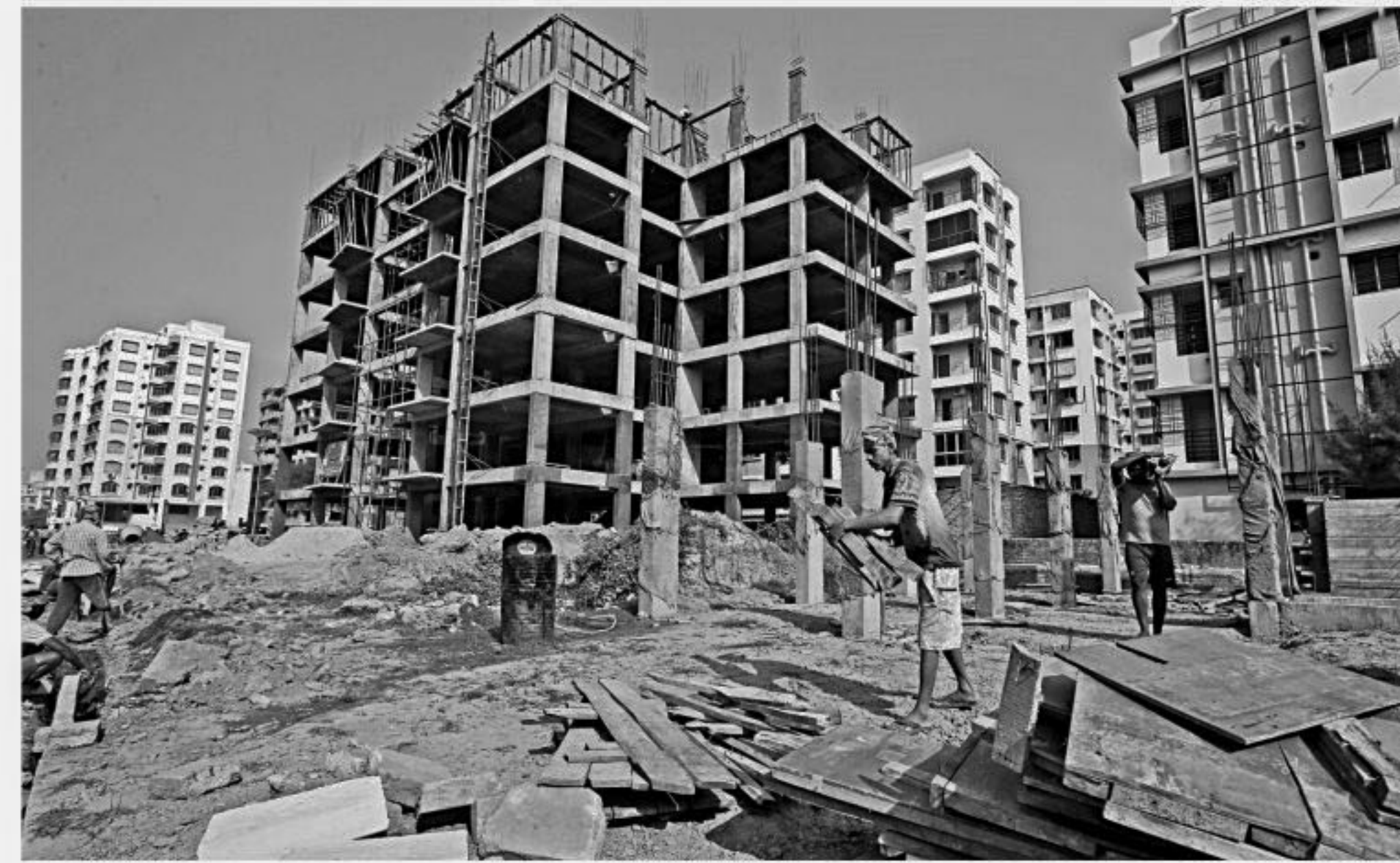
Labourers work at the construction site of residential buildings on the outskirts of Kolkata.
