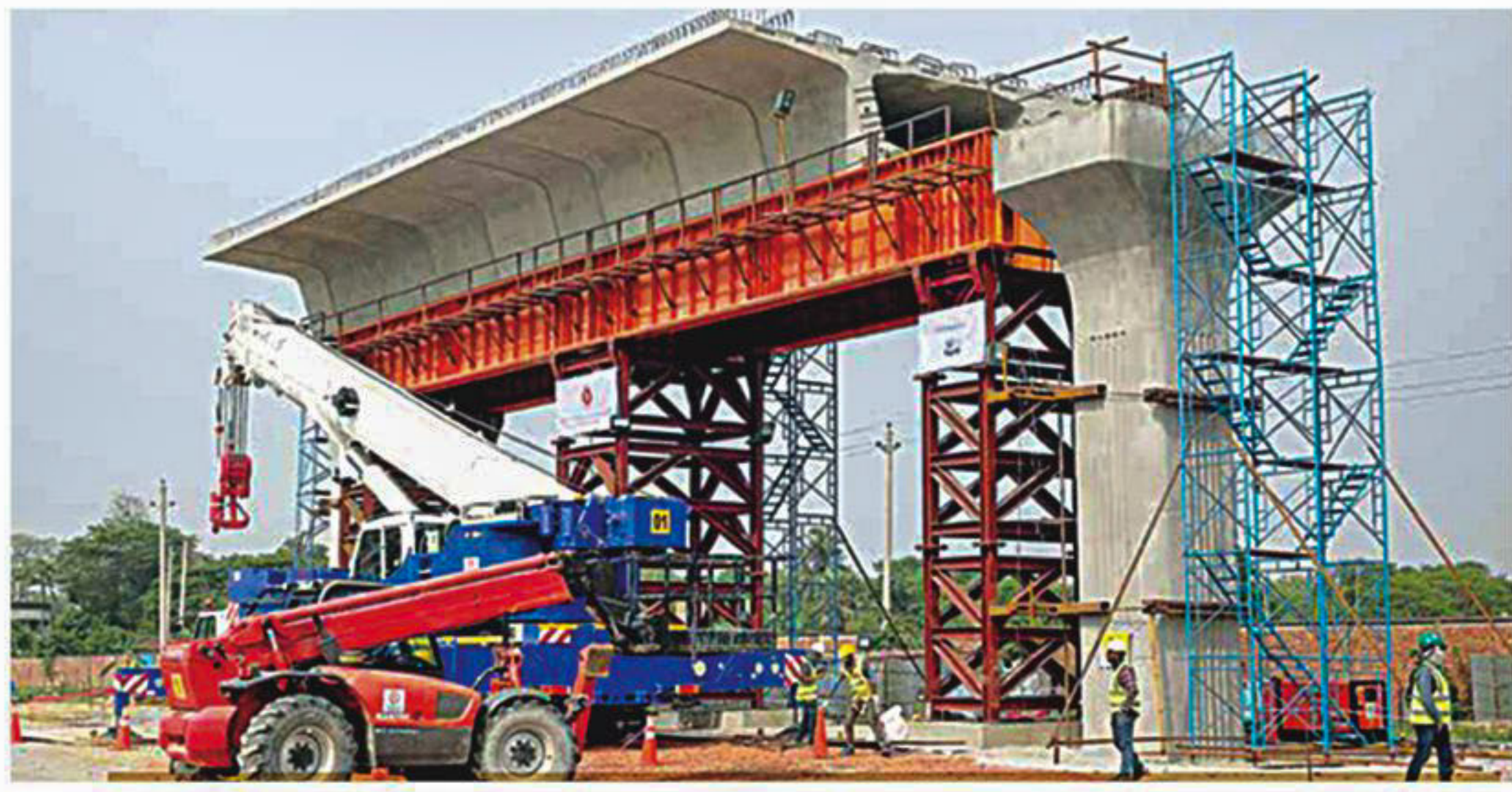
Precast box girders of Metro Rail Project are fabricated in a construction yard and transported to the site for joining together by pre-stressing steel.
