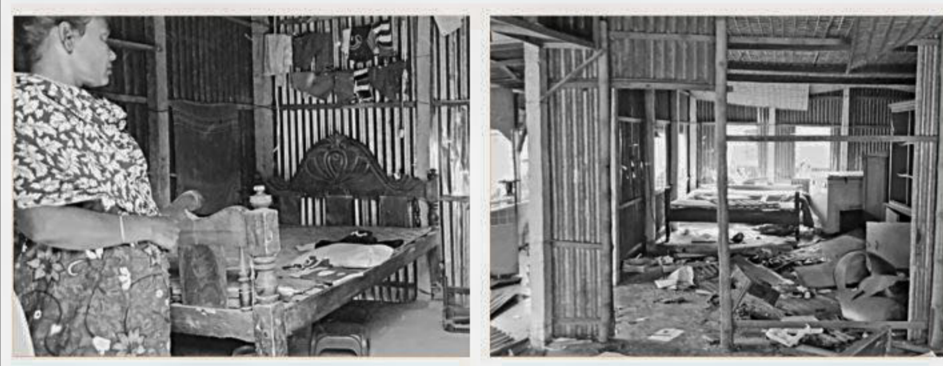
Above, villagers flee homes for safety following series of clashes between followers of two local leaders of Awami League at Bilchandak village in Pabna's Faridpur upazila on Wednesday. Below, many houses, like these ones in the picture, lie badly damaged after an orgy of vandalism for three consecutive days. PHOTO: AHMED HUMAYUN KABIR TOPU
