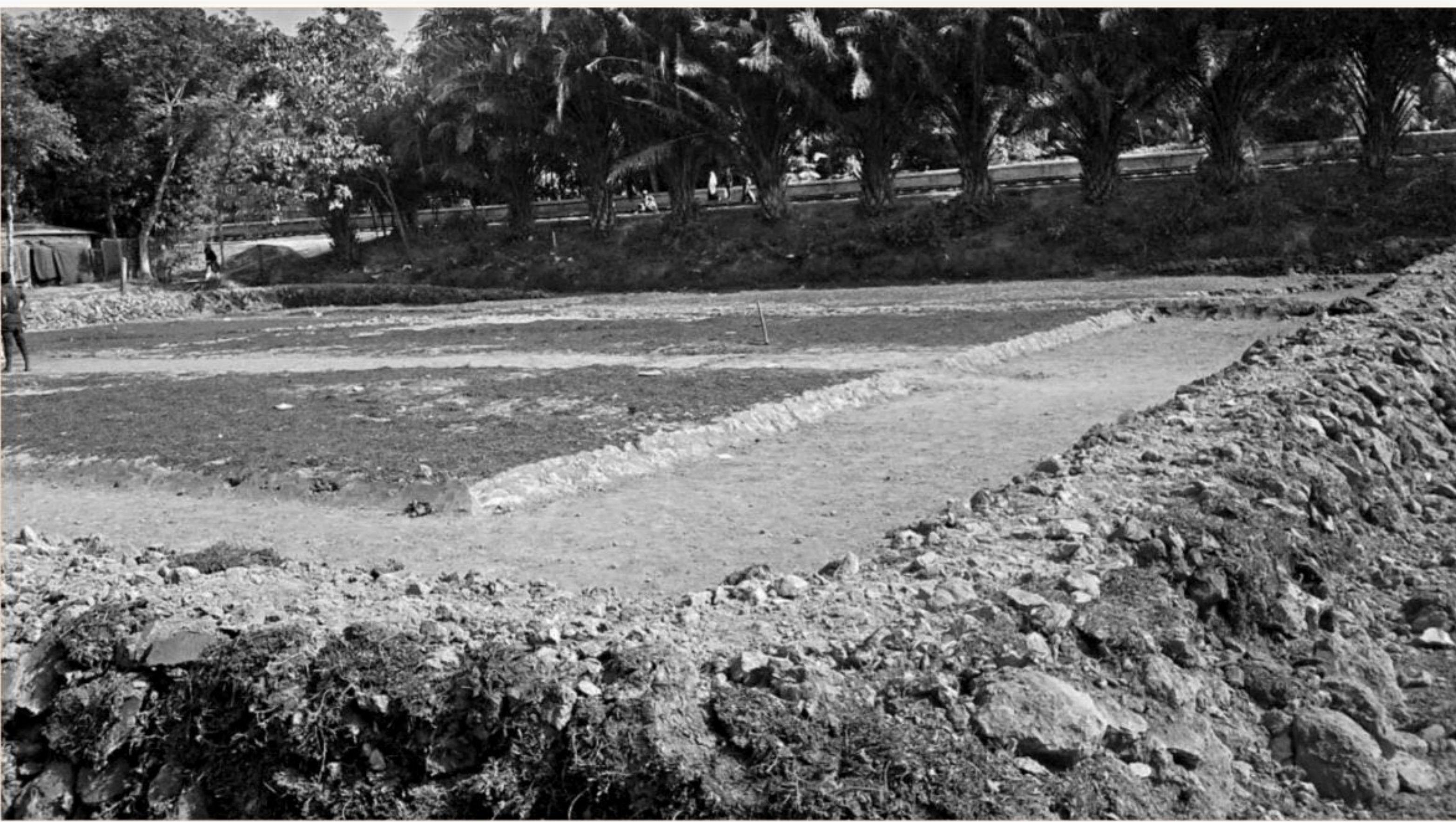
Workers engaged by a local influential person have continued digging a pond illegally on 10 decimals of land belonging to Bangladesh Railway in Kamalganj upazila of Moulvibazar.
