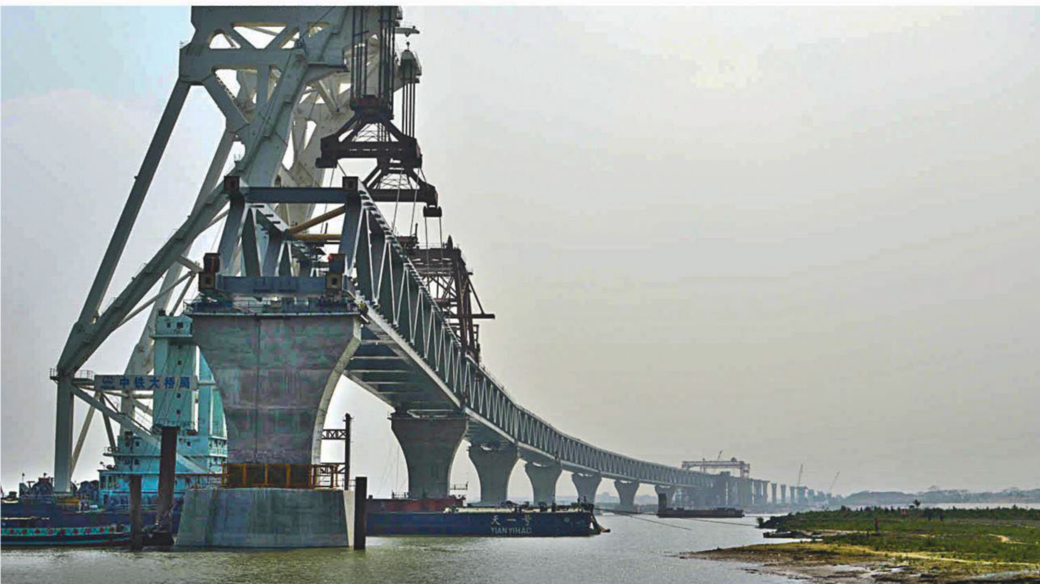
The eighth span (superstructure) of the under-construction Padma bridge was installed at Jajira point of Shariatpur yesterday, making about 1,200 metres of the 6.15-kilometre megastructure visible. The latest 150-metre span was placed on pillars 35 and 36.
