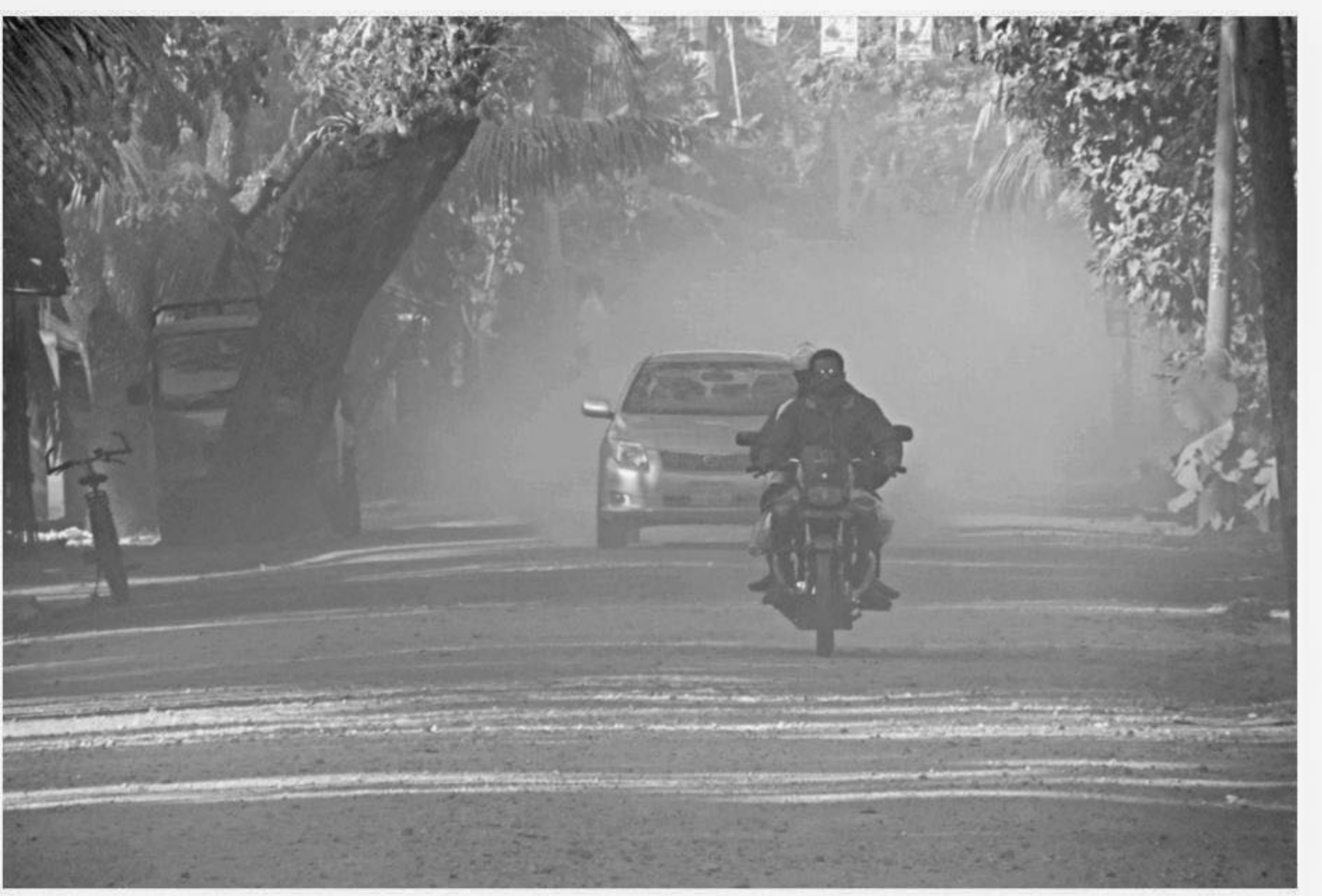
Thick dust blurs vision and poses health hazard for commuters and locals as the menace turns serious on an 18-kilometre stretch of road from Baraibari to Kanudaskathi in Jhalakathi amid the ongoing road reconstruction work, being done with little remedial measures like spraying of water. The photo was taken from Brac More area of Jhalakathi a few days ago. PHOTO: STAR
