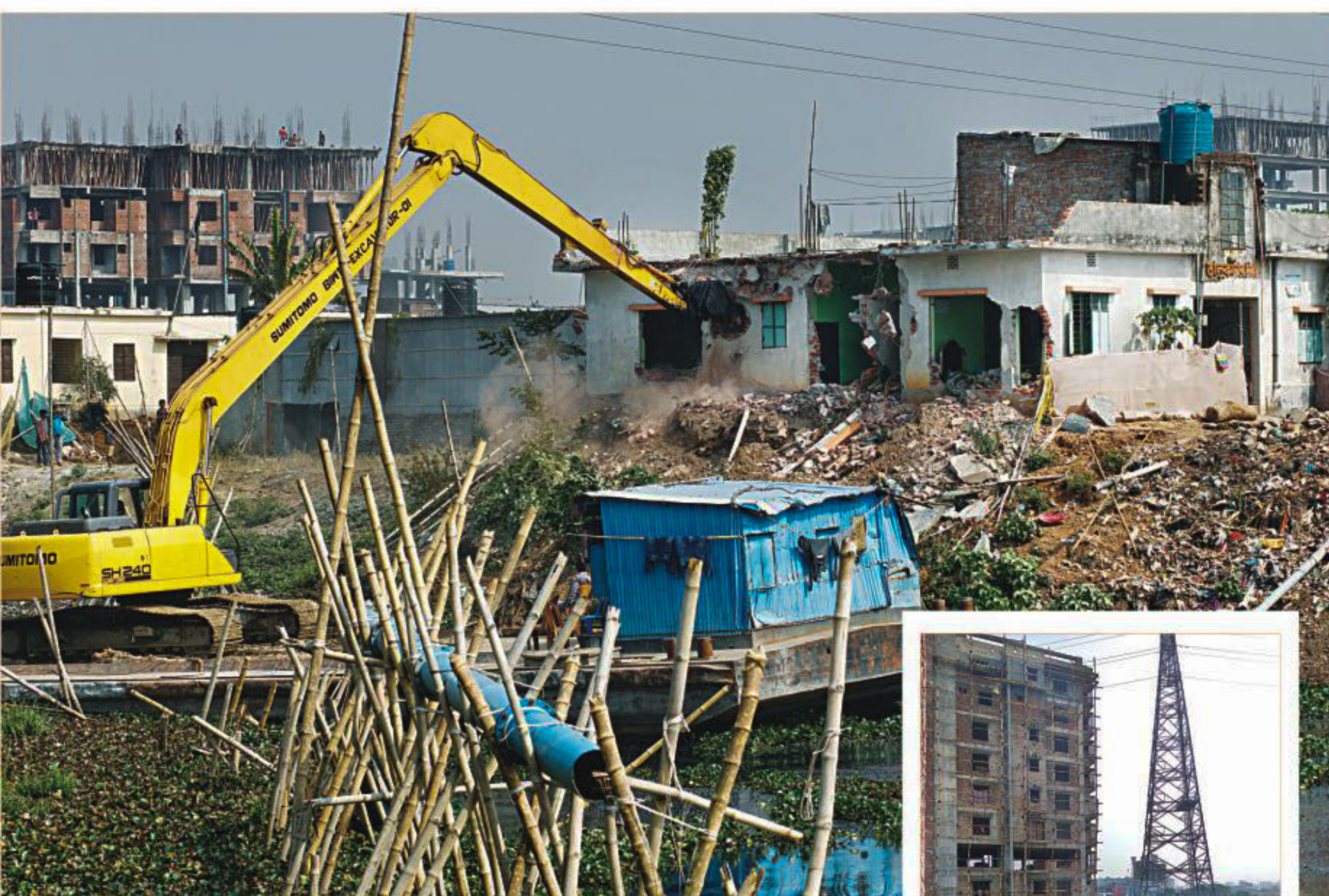
A bulldozer demolishes a building on the bank of the Buriganga river in Bosila area of the capital during a BIWTA drive against encroachers yesterday morning. Inset, a building left unscathed while the surrounding ones have been razed.
