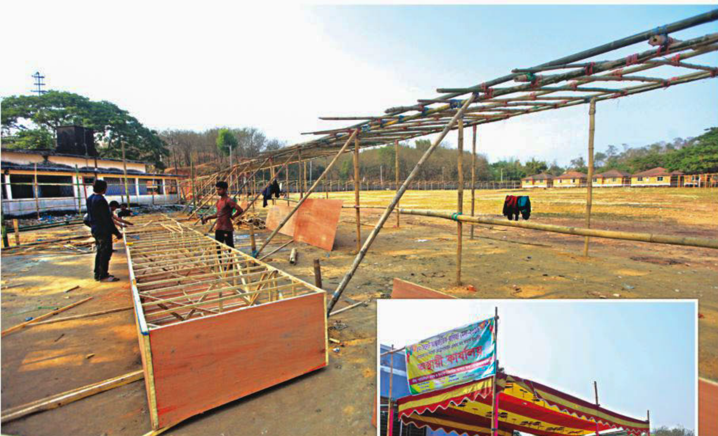
Barely a month has passed since the last trade fair ended at Sheikh Russel Mini Stadium in Sylhet. Now, work is going on to hold another month-long fair. Inset, a temporary office set up by organisers.
