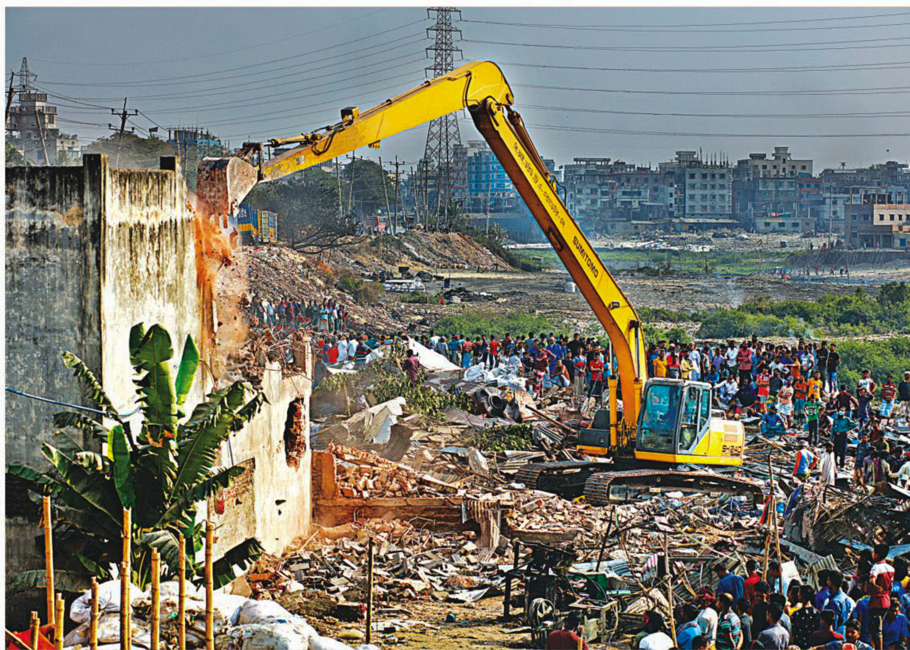
A bulldozer demolishes an illegal structure on the Buriganga during an eviction drive by the BIWTA in the city's Lalbagh area yesterday. The authorities carried out the drive to save the river from encroachment. Story on page 2.
