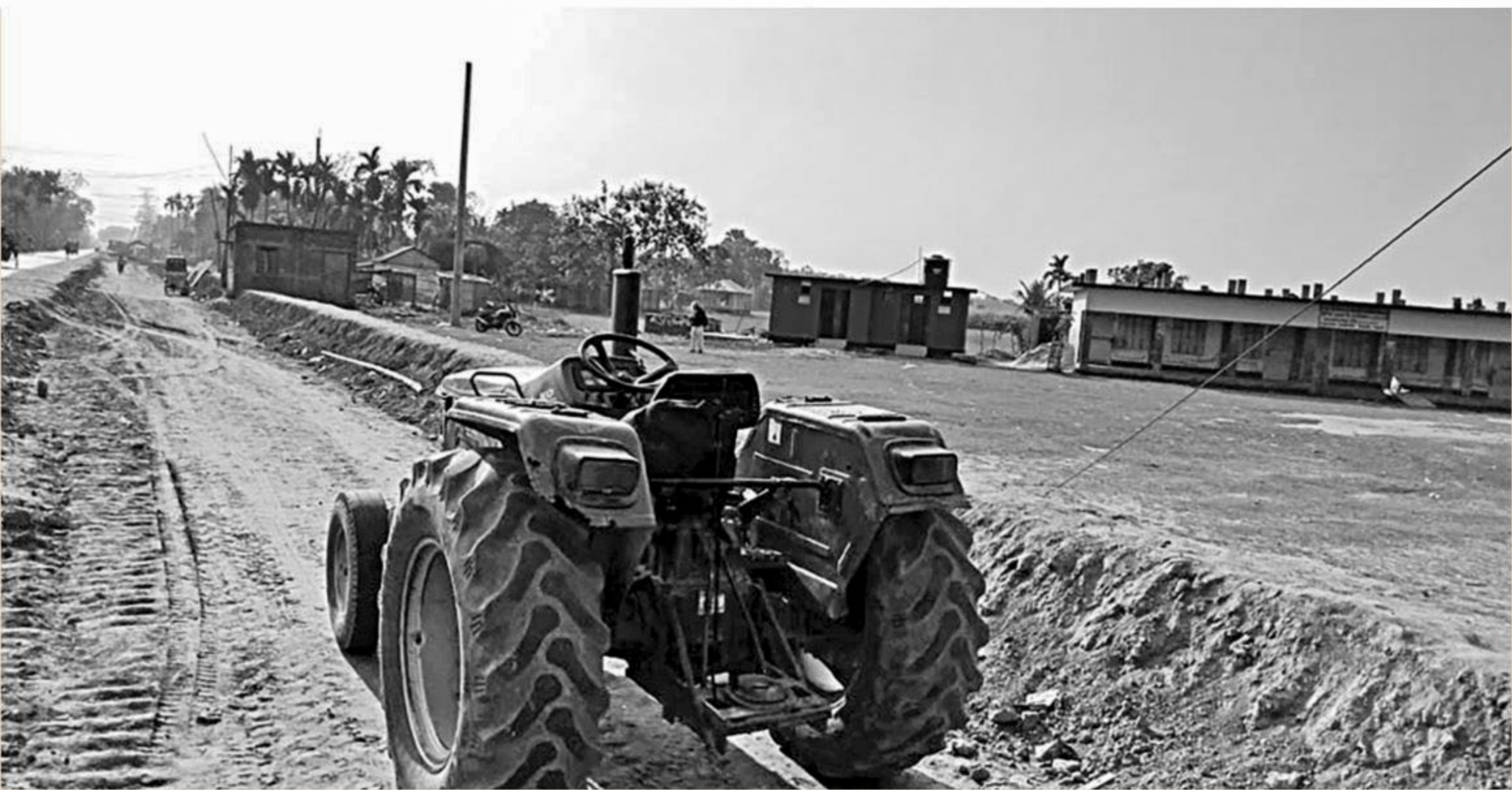
Work for a railway line has started just in front of two schools (one not in picture) beside Ishwardi-Rooppur road at Sara Gopalpur village in Ishwardi upazila of Pabna, giving rise to safety concerns among teachers, students and guardians.
