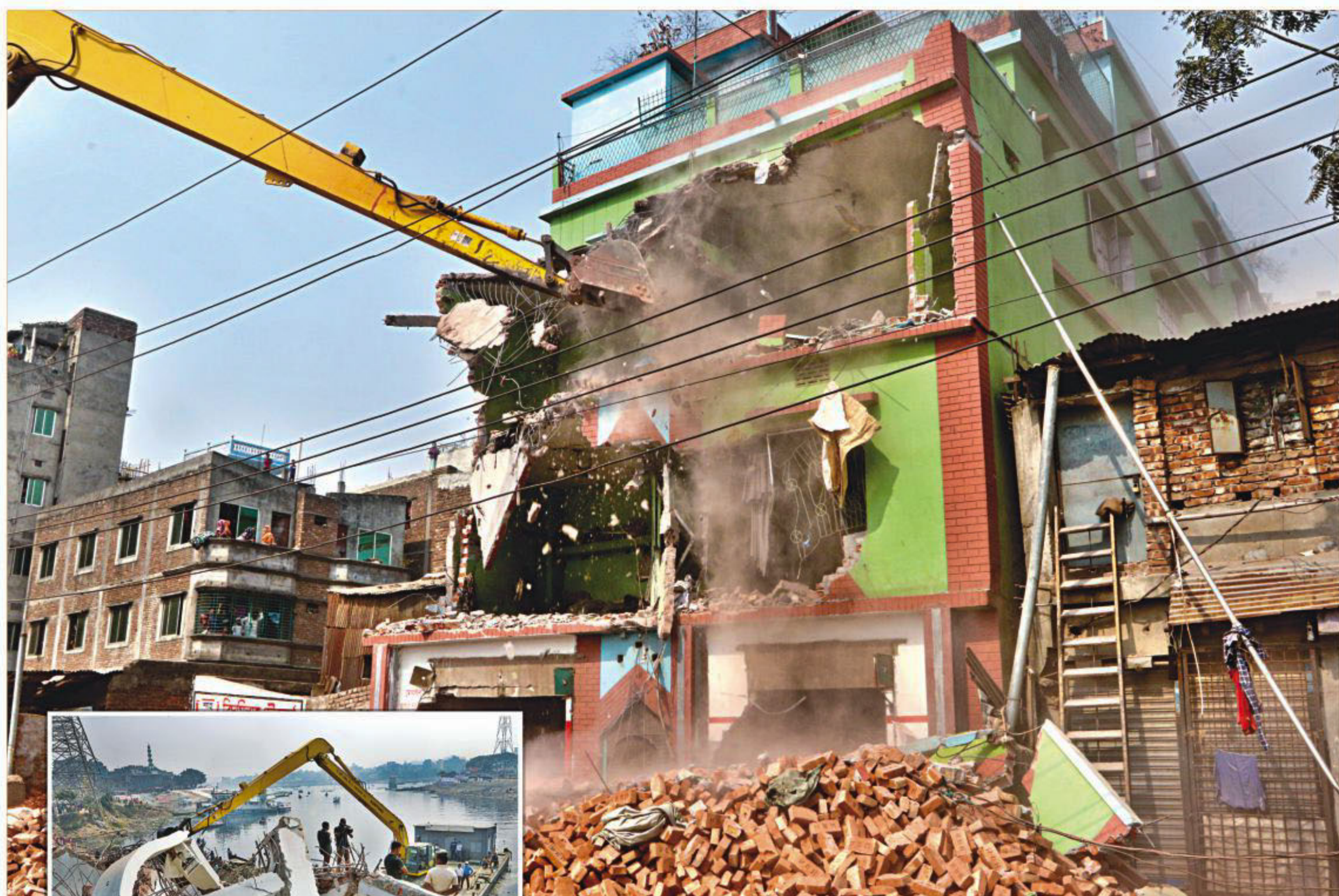
The arm of an excavator wrecking a building at Islambagh in the capital's Kamrangirchar by the Buriganga river during a drive conducted by the Bangladesh Inland Water Transport Authority against encroachers yesterday.
