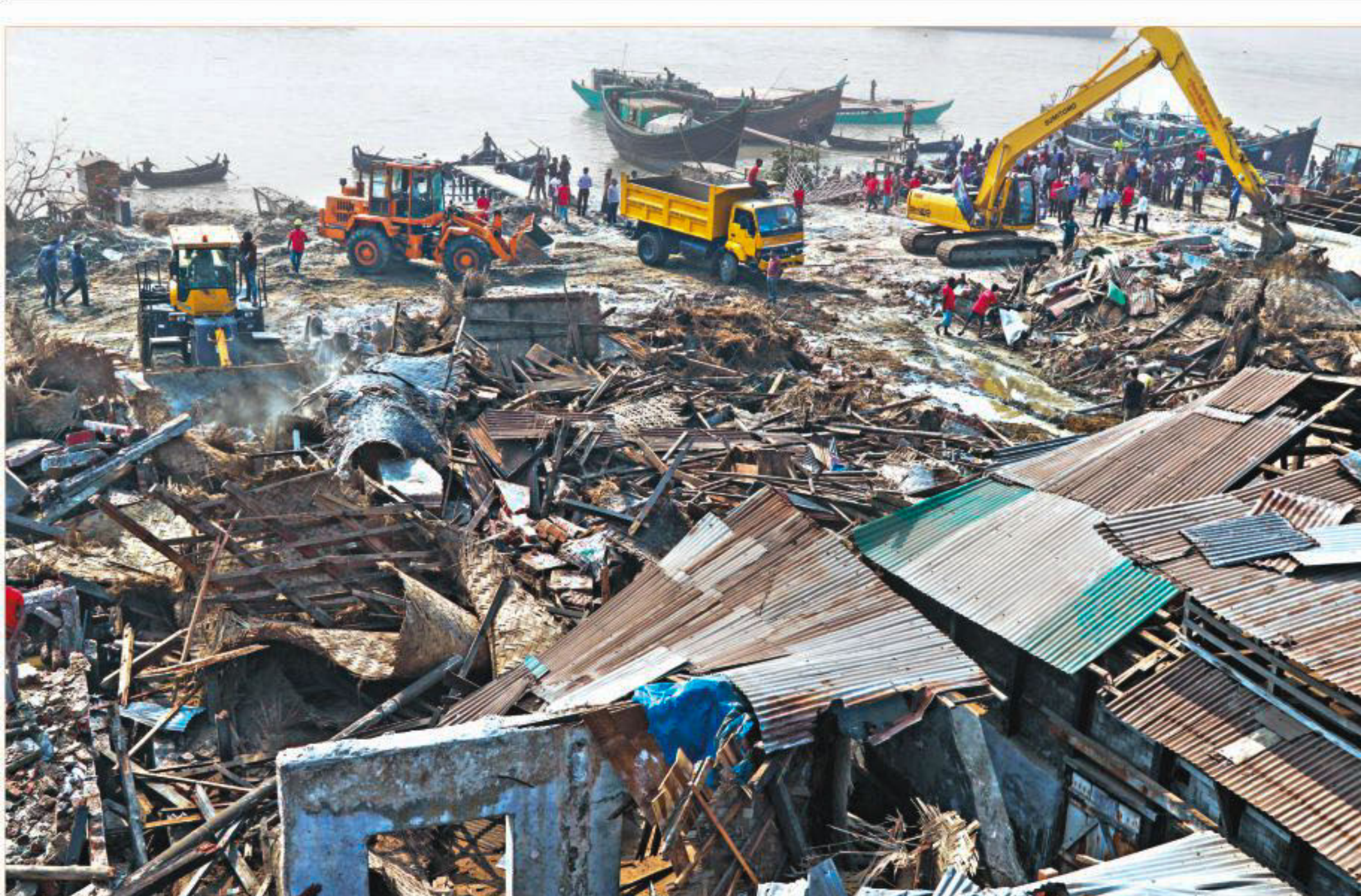
Erection drive continues on Karnaphuli river banks. On the third day, 40 structures were demolished, bringing the total number of dismantled structures to 120.
