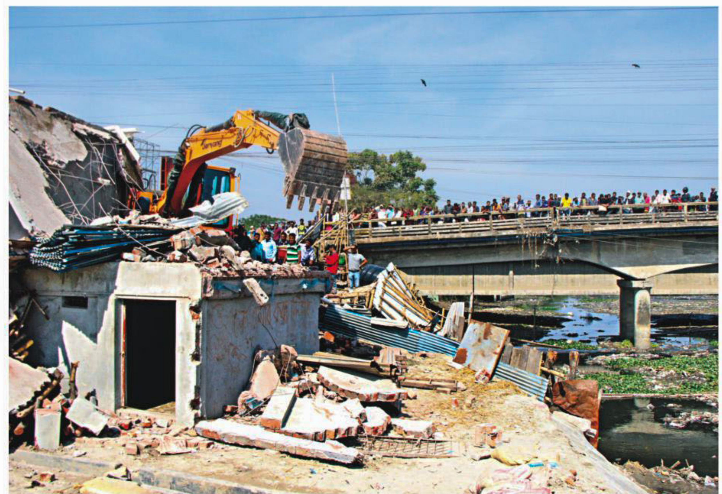
An excavator ploughs through illegal structures along Mayur Nadi canal in the Gallamari Bridge area in Khulna, as people gather to watch in the distance.
