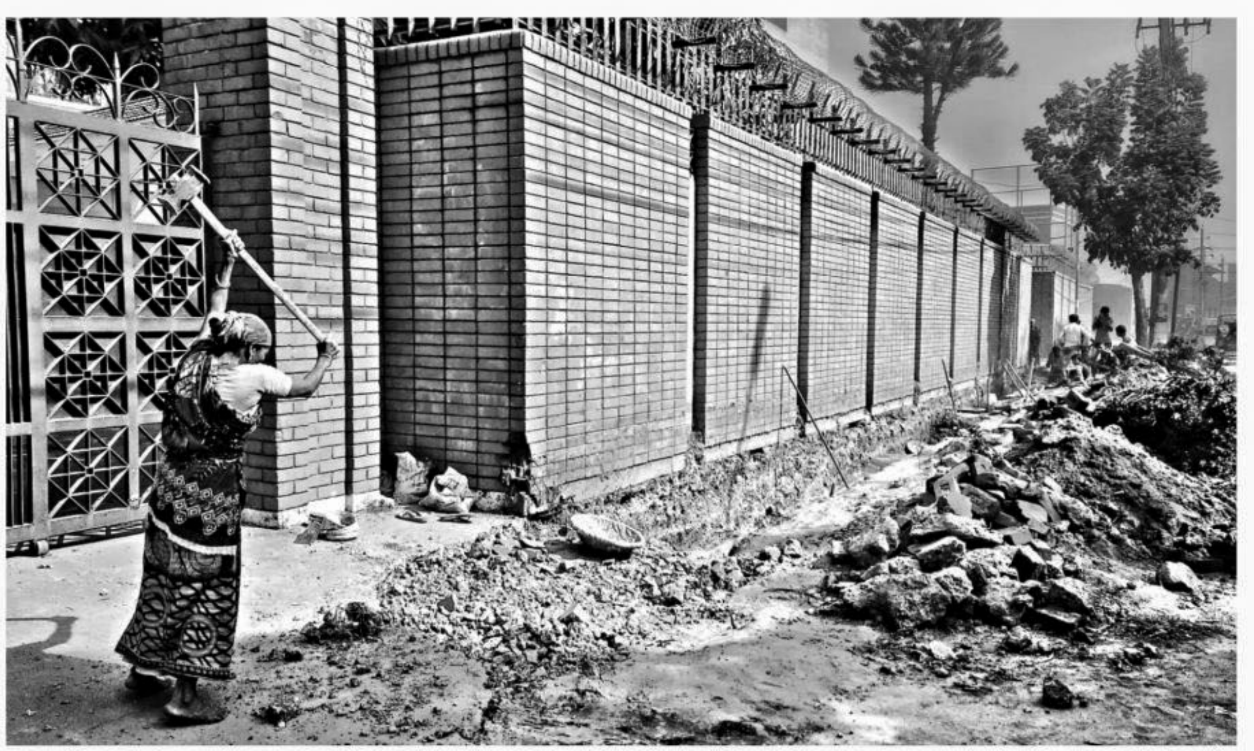
A labourer takes her heels off the ground as she musters all her strength to wield a sledgehammer, tearing down the footpath on the Madani Avenue in the capital. Dhaka North City Corporation is digging a drain in the capital's diplomatic enclave, heaping debris on the side of the road that is obstructing pedestrians' path and causing air pollution.
