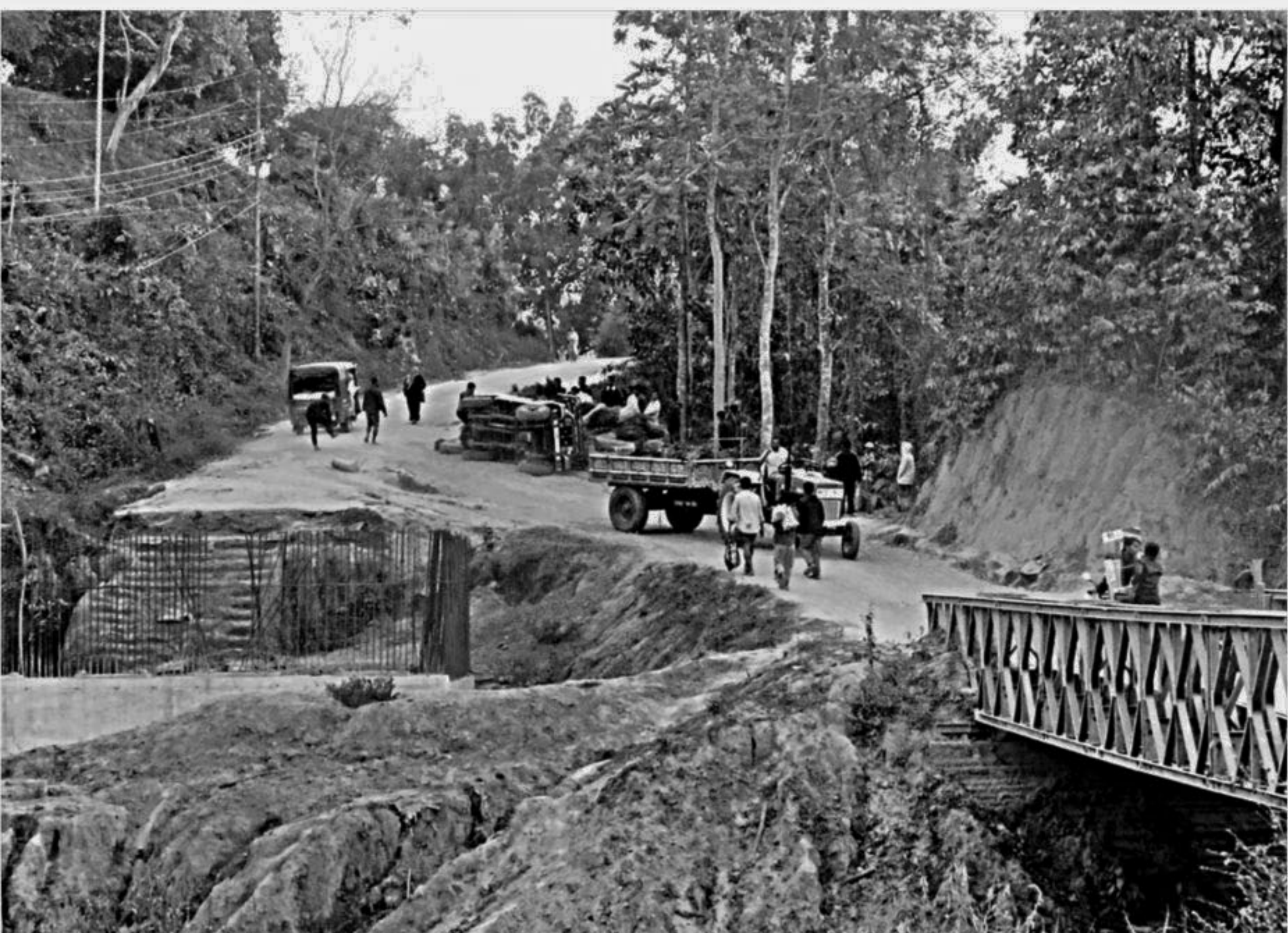
The diversion road beside Thakurchara Bridge on Khagrachhari-Mahalchhari road in Khagrachhari is lying in an awful condition, posing risk for vehicles and commuters. The spot saw several accidents including the one on Tuesday when a jeep overturned there. PHOTO: STAR
