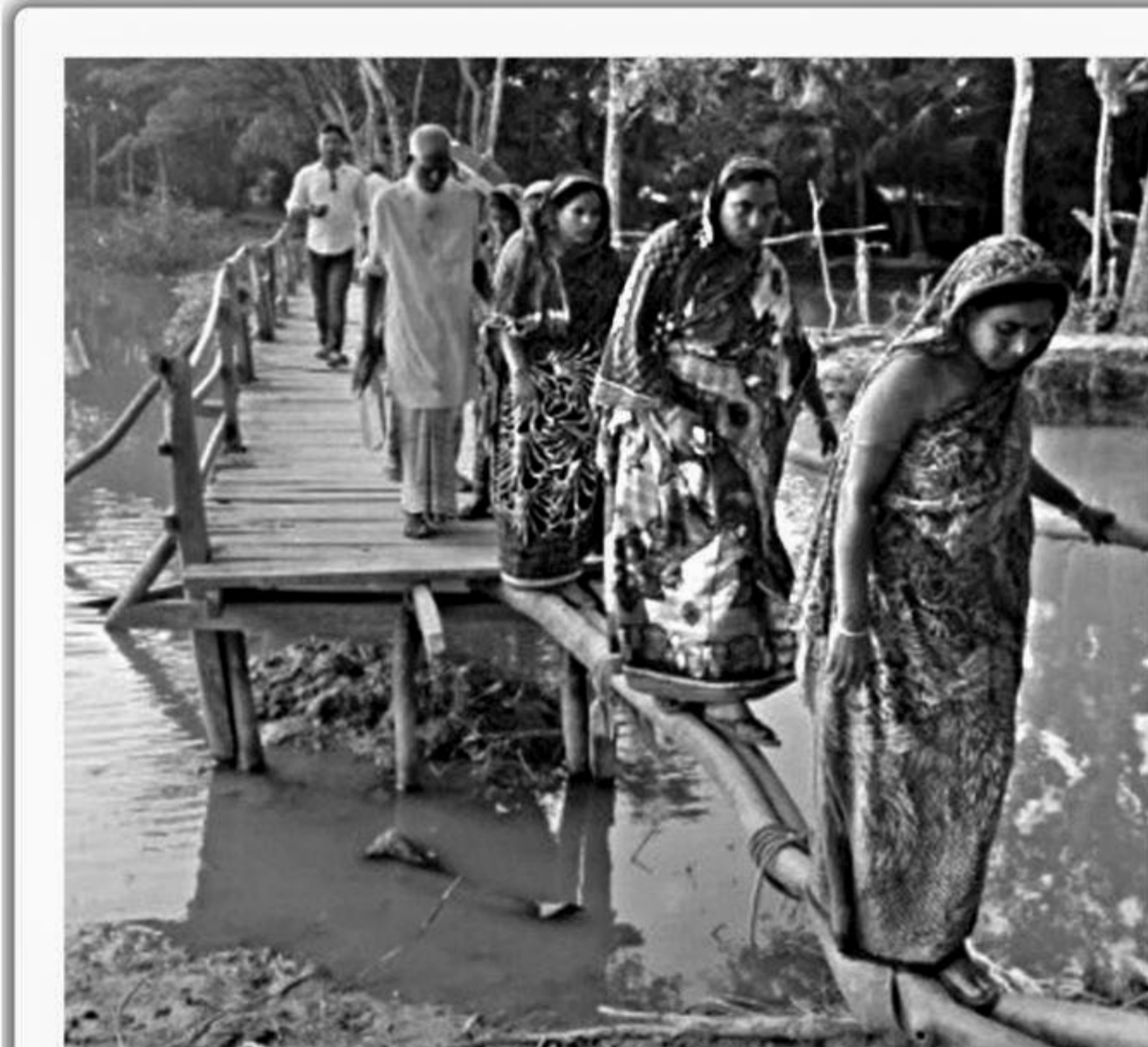
People cross with difficulty a dilapidated bridge at Charipara in Kalapara upazila of Patuakhali.
