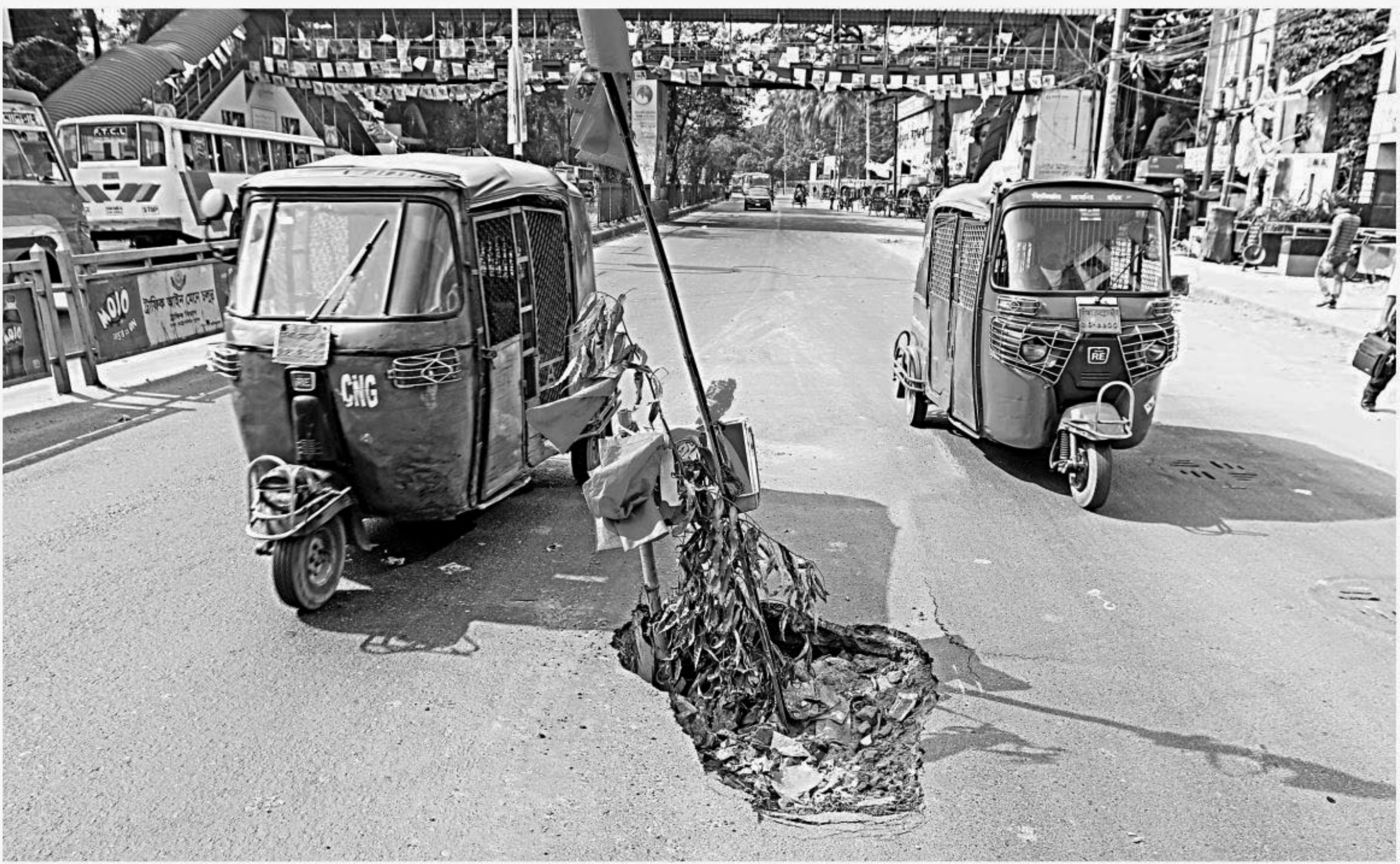
Two auto-rickshaws avoid a crater in front of Jatiya Press Club. Hundreds of vehicles have to do the same on a busy workday, causing long tailbacks, although it needs little to alleviate public suffering. The photo was taken yesterday. PHOTO: PALASH KHAN
