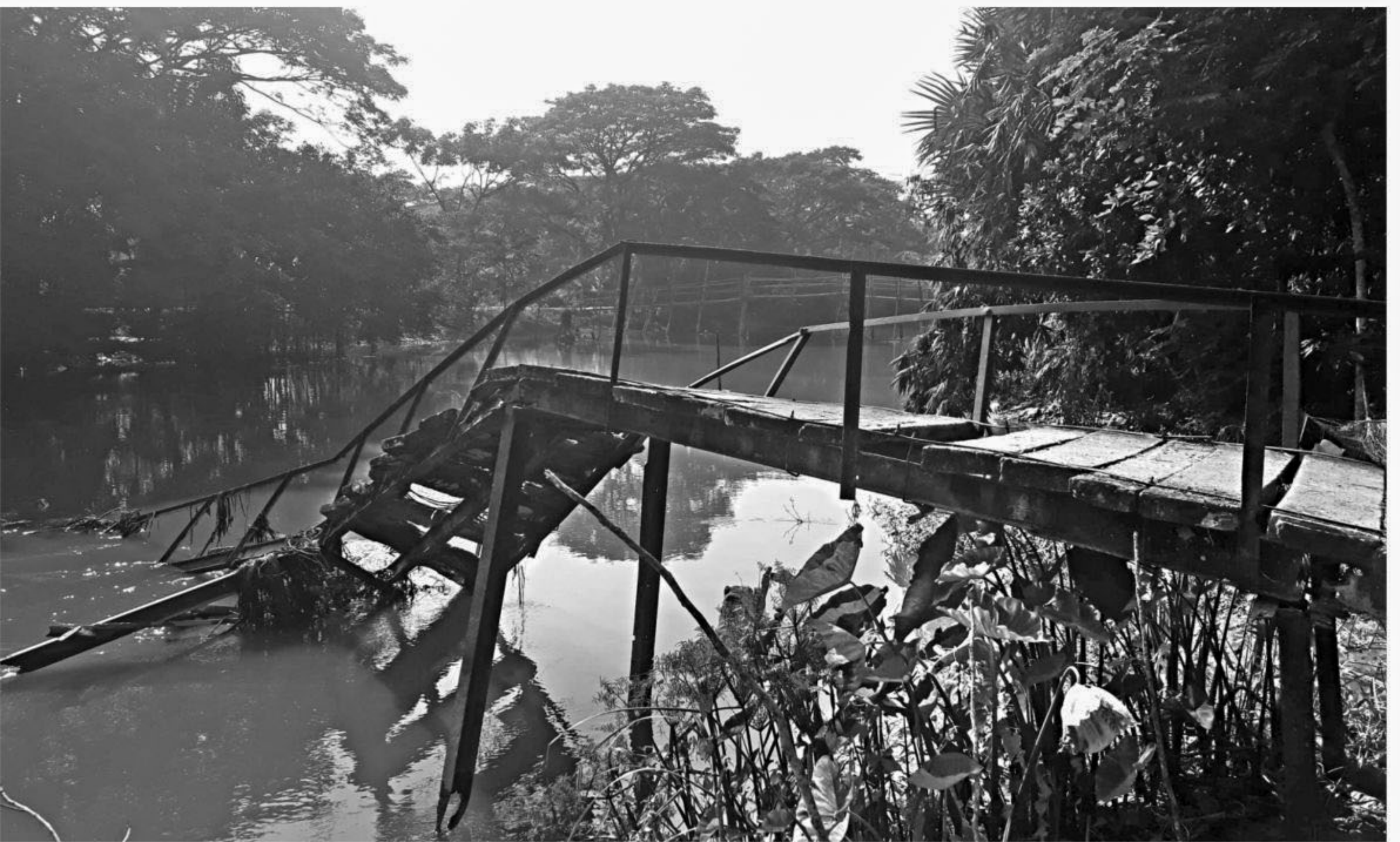
This 30-year-old iron bridge built over Bauria canal in Galachipa upazila of Patuakhali collapsed one and a half months ago.
