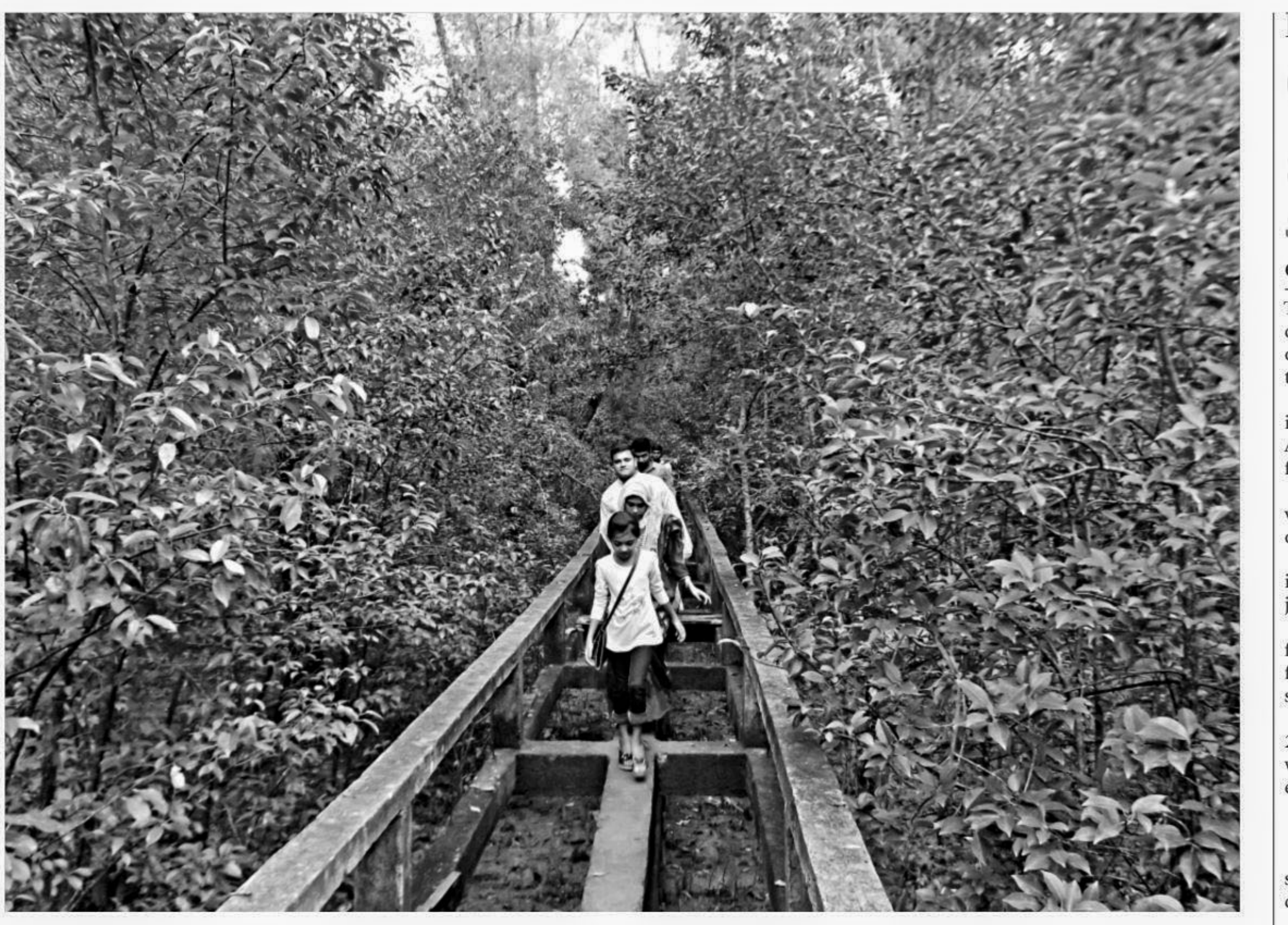
Visitors face troubles while walking through the dilapidated foot rail in Horinghata reserve forest of Pathorghata upazila in Barguna.
