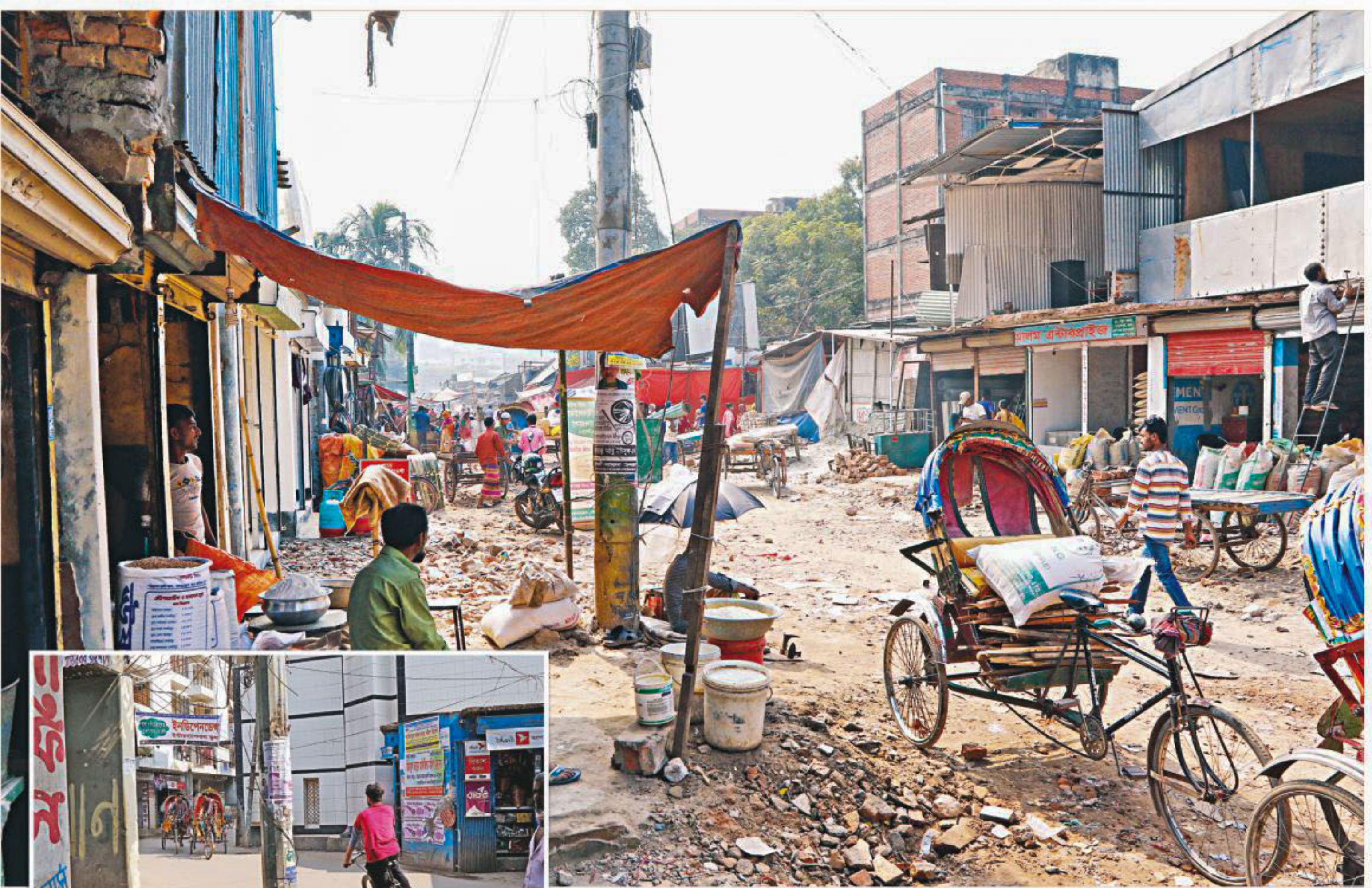
A road being extended and repaired in South Paikpara, after locals vacated space in front of their establishments. Inset, a widened road in the area. The photos were taken recently.
