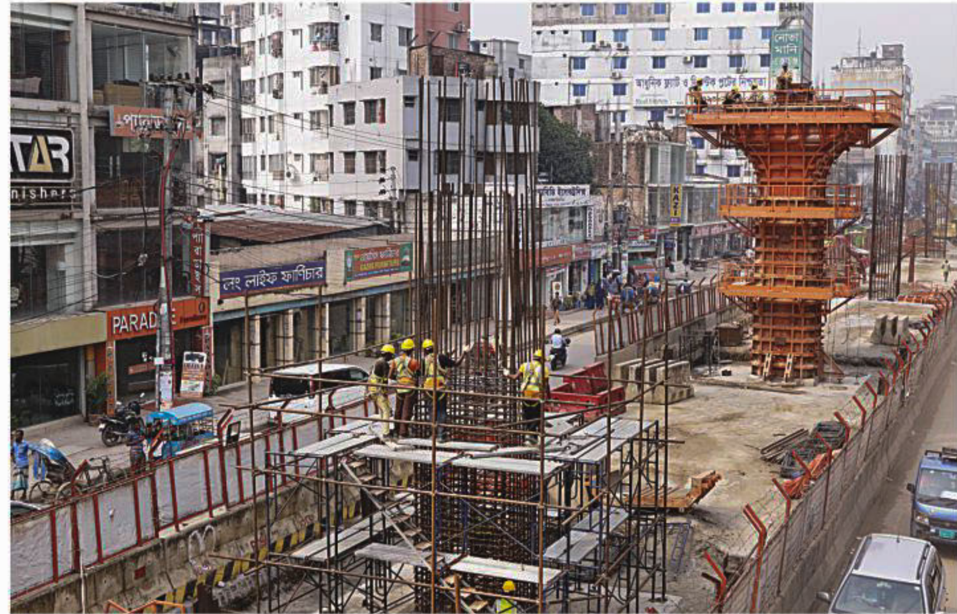
A construction site of the Dhaka Metro Rail near Rokeya Sharani. PHOTO: PALASH KHAN
