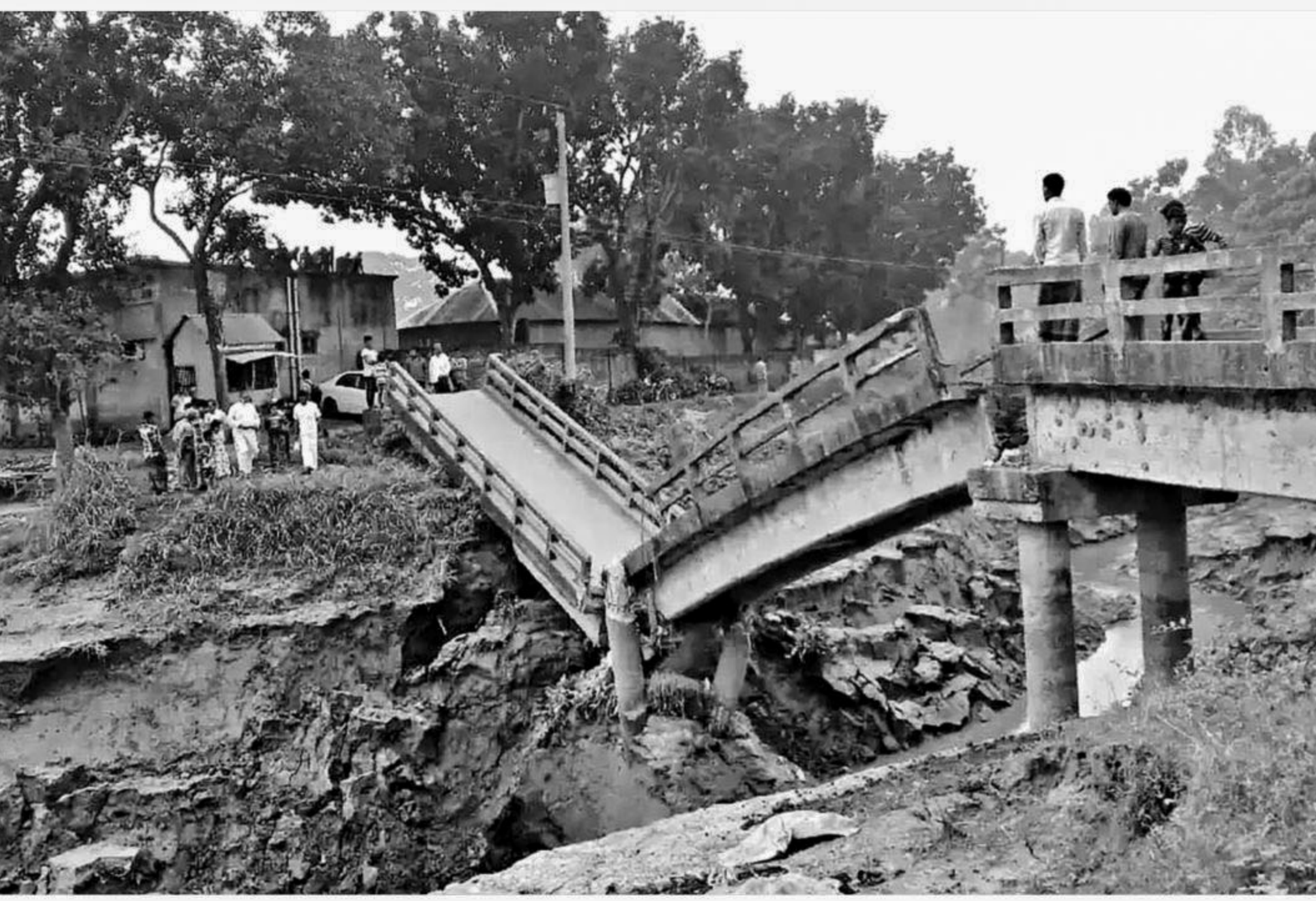
The bridge at Fotepur in Mirzapur upazila of Tangail collapsed on Wednesday as the earth under it was washed away during the last rainy season, making the structure weak.
