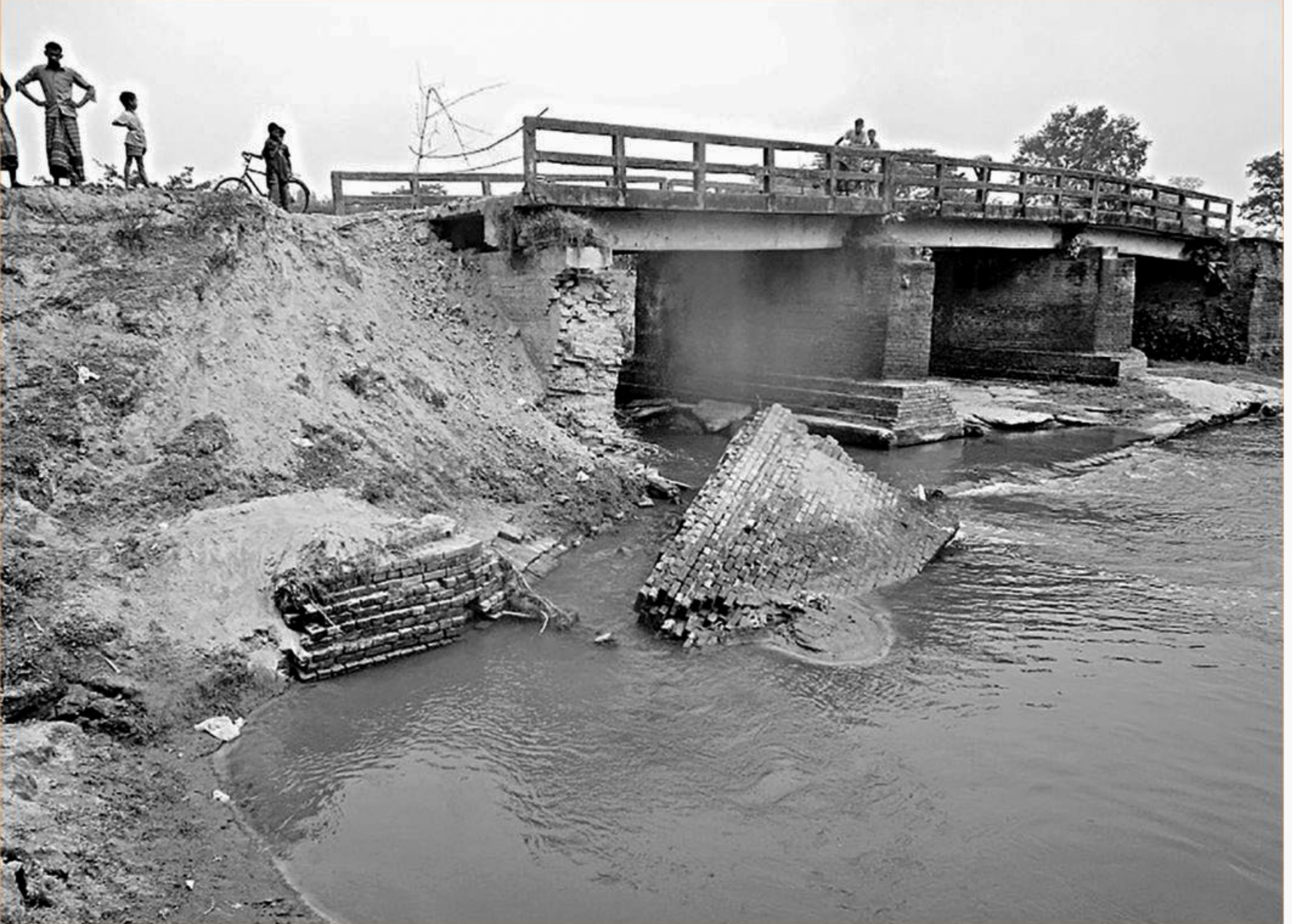
A wing wall and approach road of a bridge over the Kharuvaj river at Nekirhat village in Taraganj upazila of Rangpur collapsed during the last rainy season.
