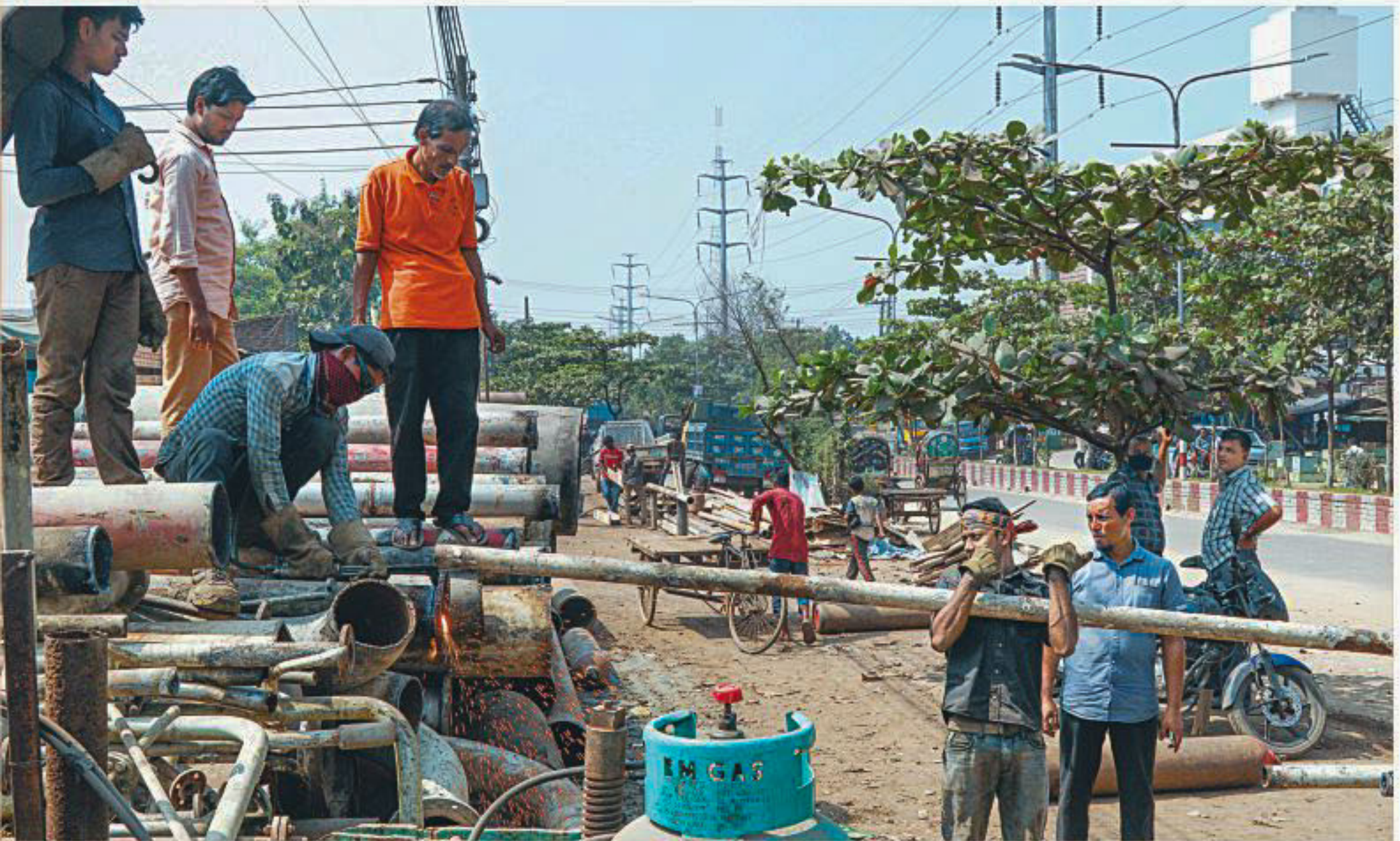
Traders occupy the entire footpath beside Sagorika Road in Chattogram city to cut scrap metals. Such a situation has been going on for years, hampering movement of pedestrians. The photo was taken at Sagorika intersection on Sunday. PHOTO: RAJIB RAIHAN
