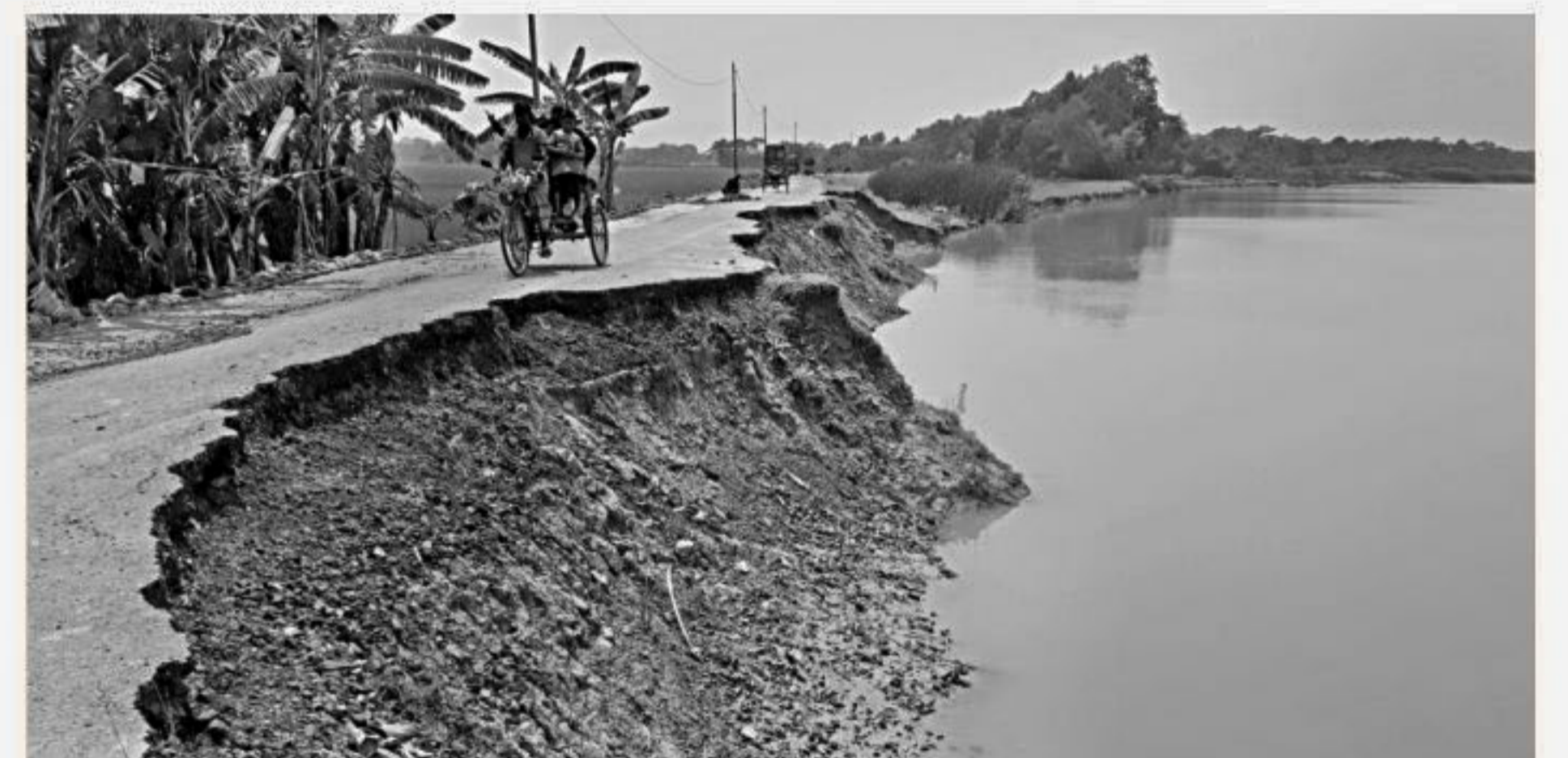
This road connecting Ronogopaldi union with Dashmina upazila headquarters has partially collapsed, leaving the locals in trouble.
