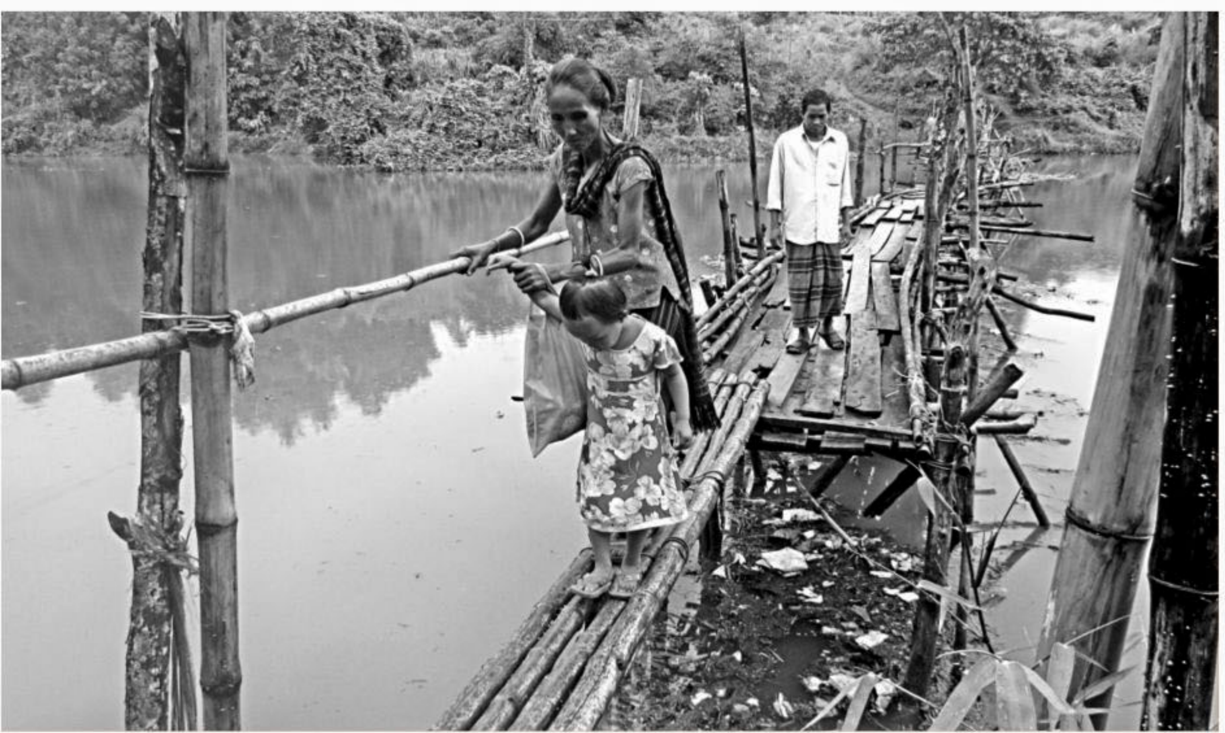
People of five villages in Rangamati municipality are suffering a lot as they have to cross this badly damaged wooden bridge in Uluchara village to go to their destinations.
