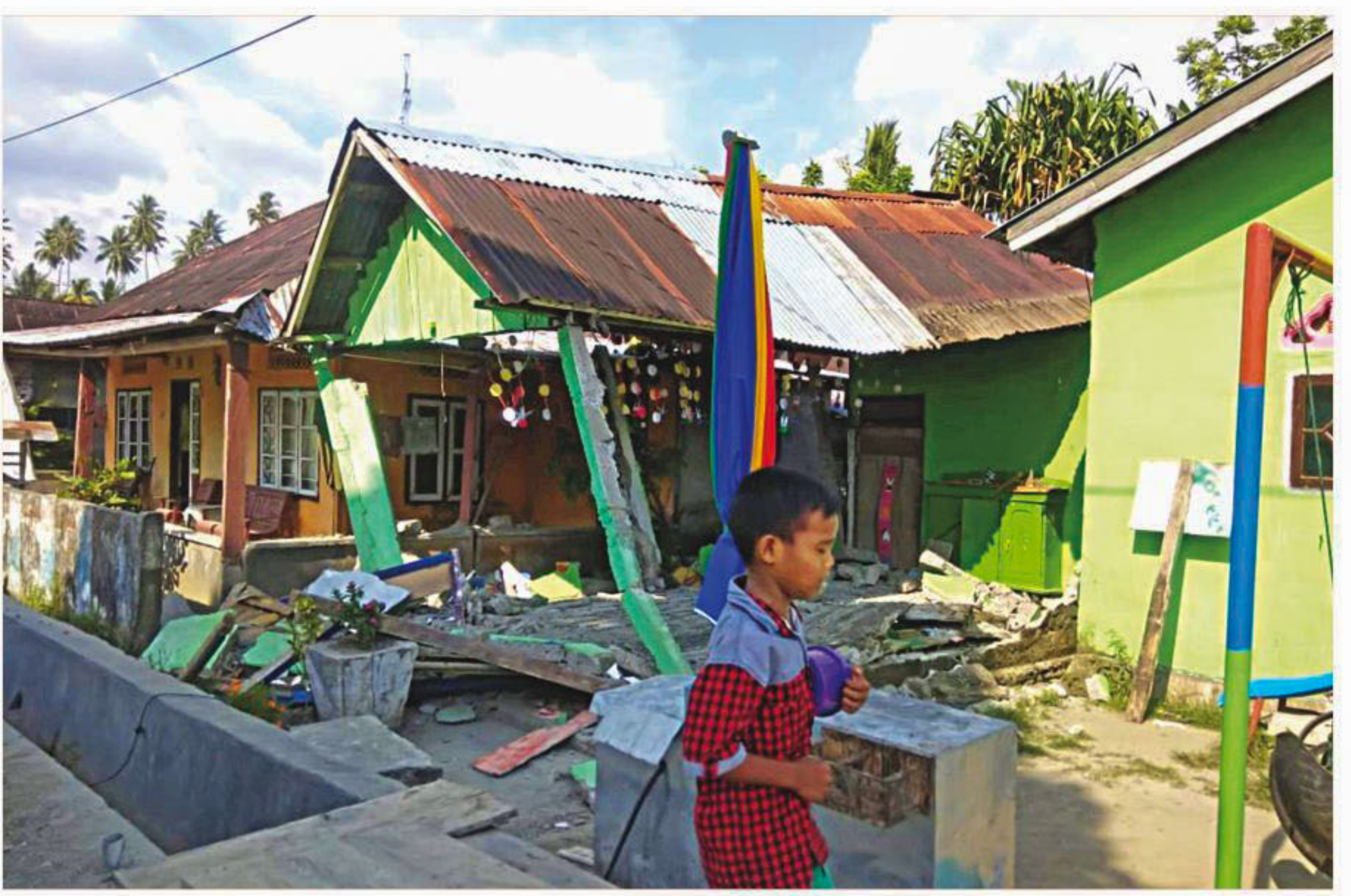
This handout photograph released by Indonesia's National Agency for Disaster Management yesterday shows a collapsed house following a powerful earthquake in Donggala, Central Sulawesi. The quake caused a tsunami that slammed into the city on Sulawesi island with officials saying the tremor had levelled many buildings. PHOTO: AFP
