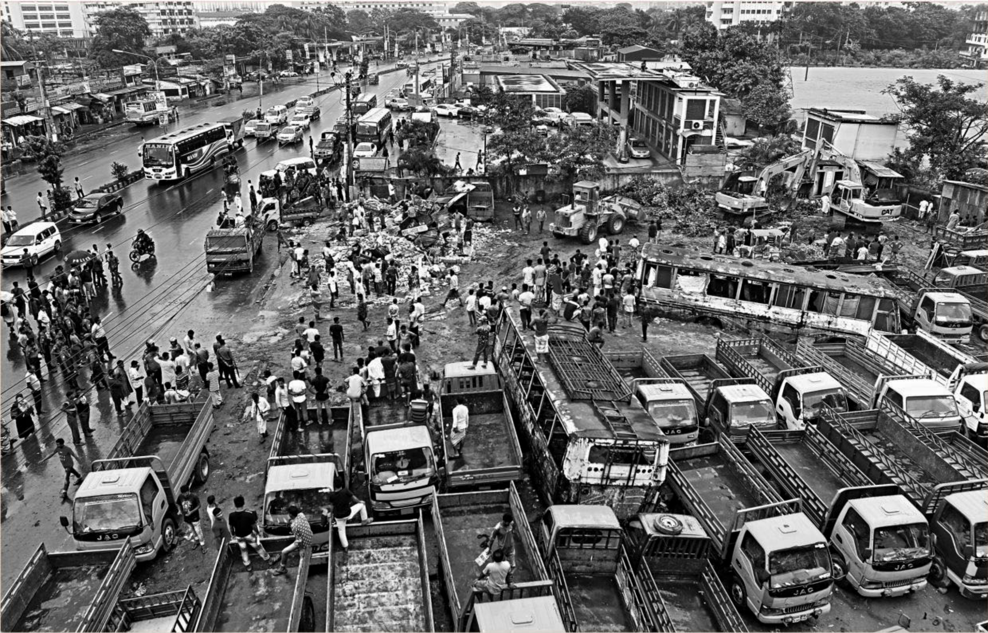
As part of a drive by the Roads and Highways Department, illegal structures are being demolished and illegally parked vehicles removed on the government land beside Mirpur Road in Gabtoli. The land will be used for the metro rail project.
