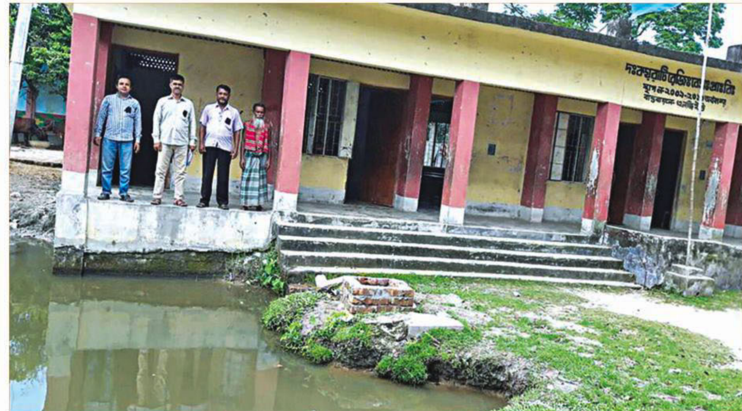
Teachers and staff at the veranda of Dakhin Koirati Government Primary School which is under threat of collapse due to landslide.
