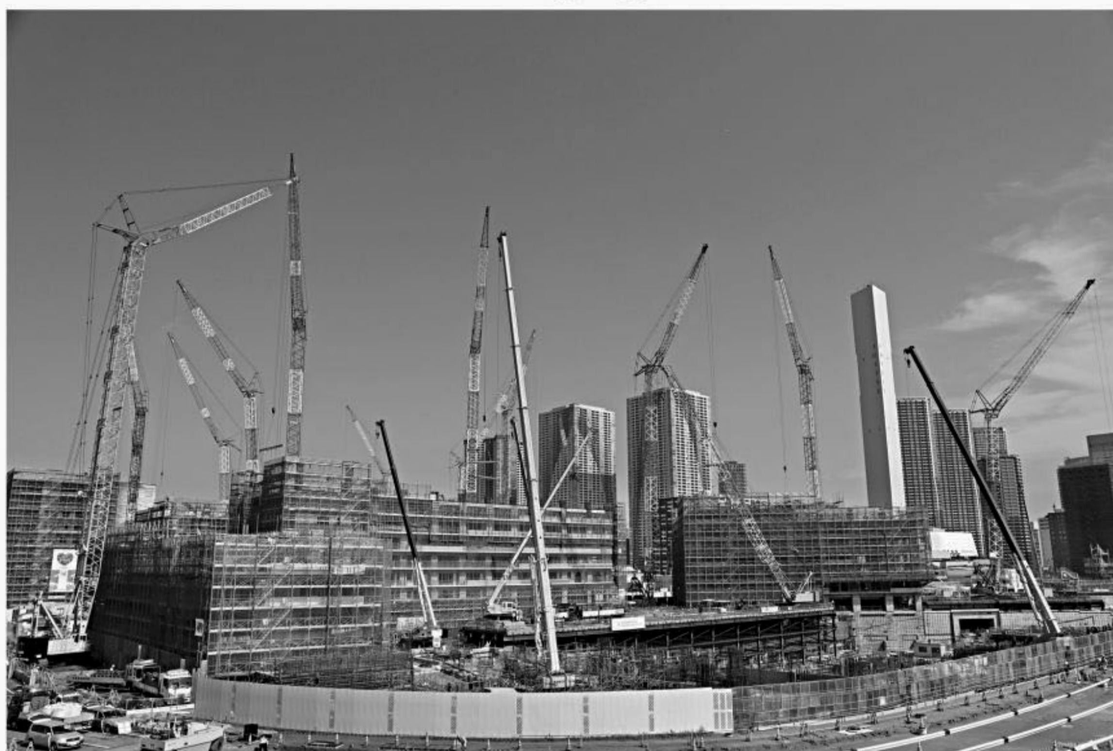
A general view of the construction site of Athletes' Village for Tokyo 2020 Olympic games in Harumi, Japan.
